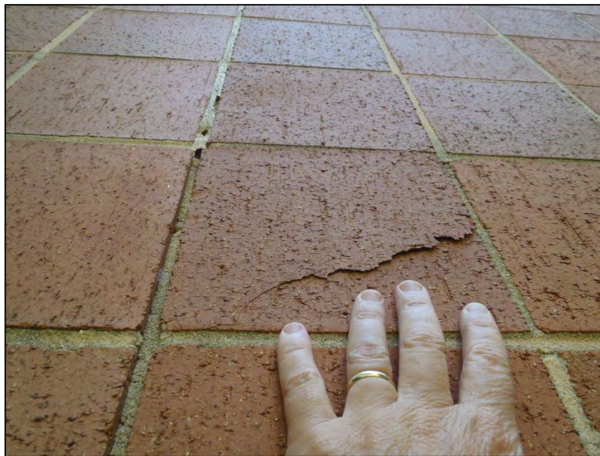
NO. 35 – EAST ELEVATION – CRACKED INDIVIDUAL MASONRY UNIT
