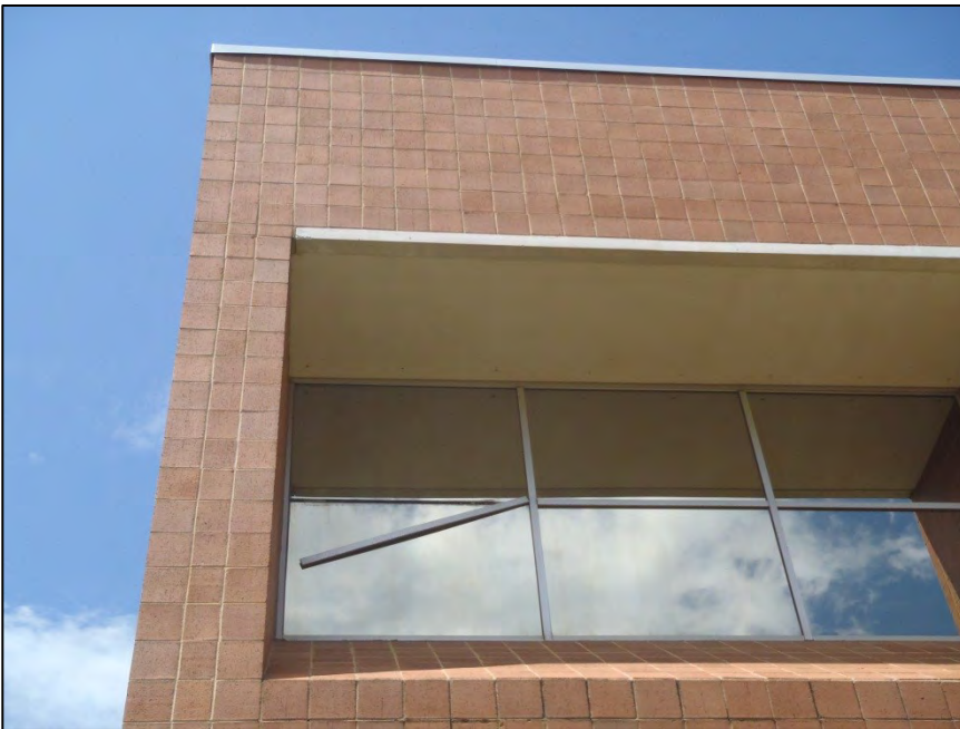
NO. 85 – SOUTH ELEVATION – DISPLACED WINDOW FRAMING
