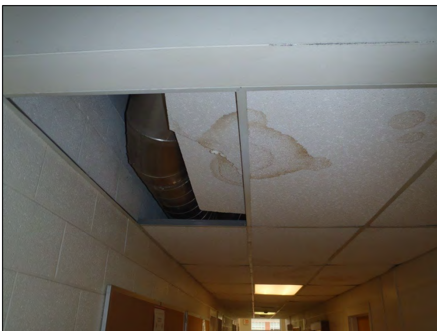
NO. 137 – SECOND FLOOR CORRIDOR – DAMAGED CEILING TILES FROM WATER INFILTRATION
