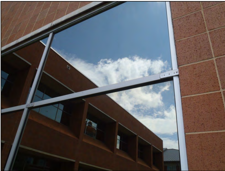
NO. 92 – SOUTHWEST ELEVATION – DISPLACED WINDOW FRAMING
