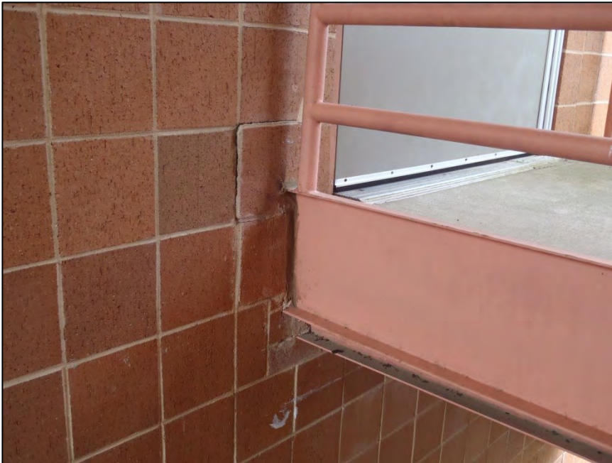
NO. 62 – NORTH ELEVATION AT CENTER EXTERIOR STAIRWELL – DETERIORATED STEEL GIRDER AND SPALLED BRICK VENEER AT BEAM BEARING LOCATION
