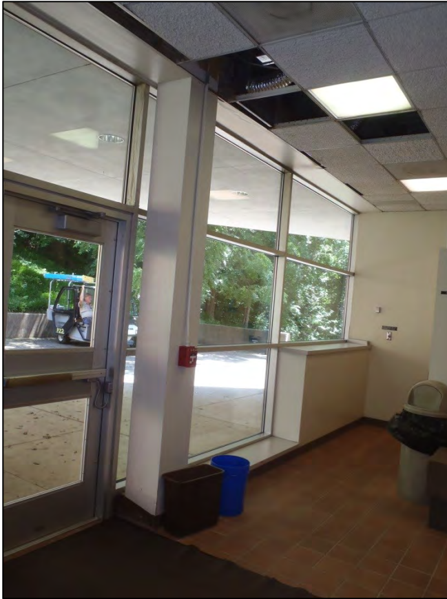
NO. 101 – FIRST FLOOR AT SOUTHEAST ENTRY PLAZA – WATER INFILTRATION
