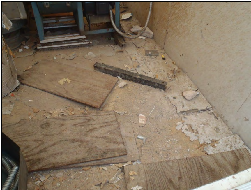
NO. 214 – ROOF SKYLIGHT/MECHANICAL ENCLOSURE – WATER DAMAGED INTERIOR FINISHES
