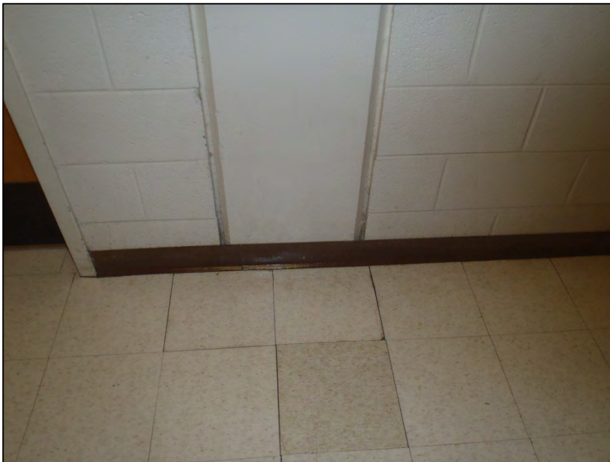
NO. 112 – FIRST FLOOR INTERIOR HALLWAY – DETERIORATED INTERIOR JOINT SEALANTS
