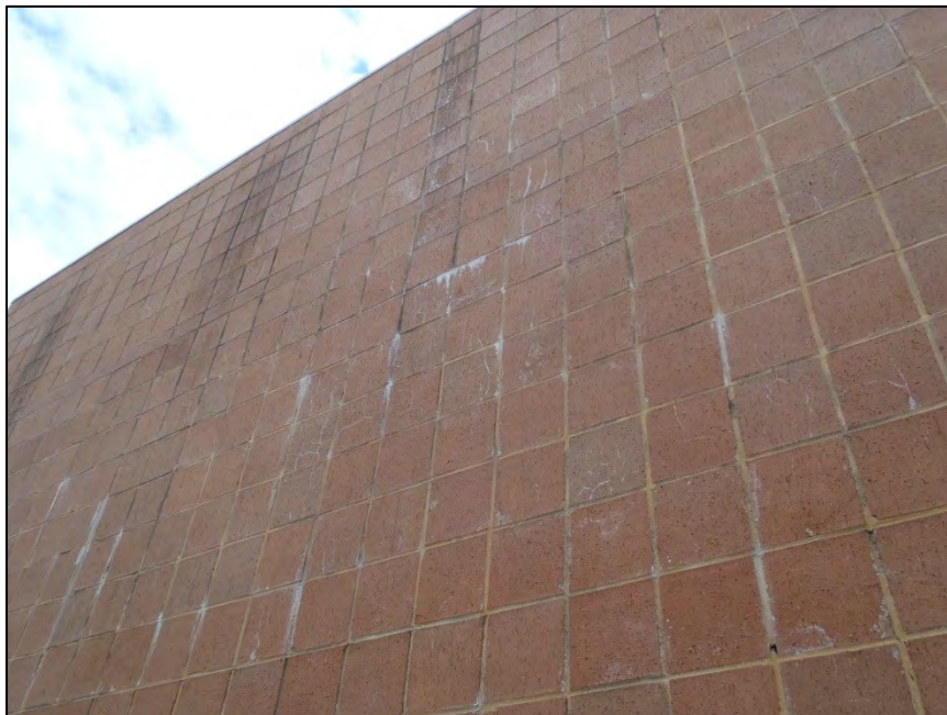
NO. 52 – NORTH ELEVATION AT EXTERIOR SCREEN WALL – EFFLORESCENCE AT EXTERIOR BRICK VENEER
