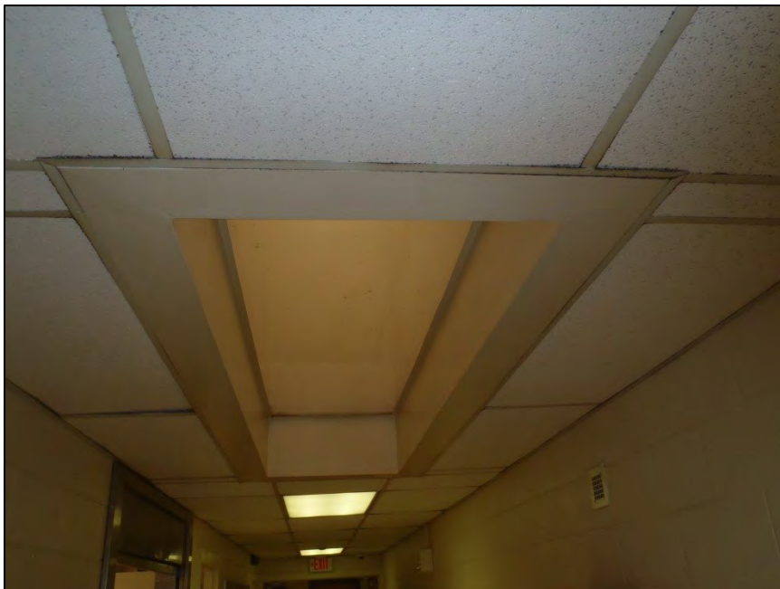
NO. 156 – SECOND FLOOR CORRIDOR – WATER STAINED SKYLIGHT DUE TO WATER INFILTRATION
