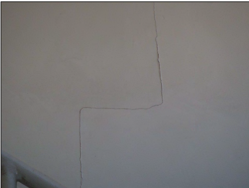
NO. 124 – SECOND FLOOR STAIRWELL AT MAIN ENTRANCE – CRACKED INTERIOR CONCRETE MASONRY
