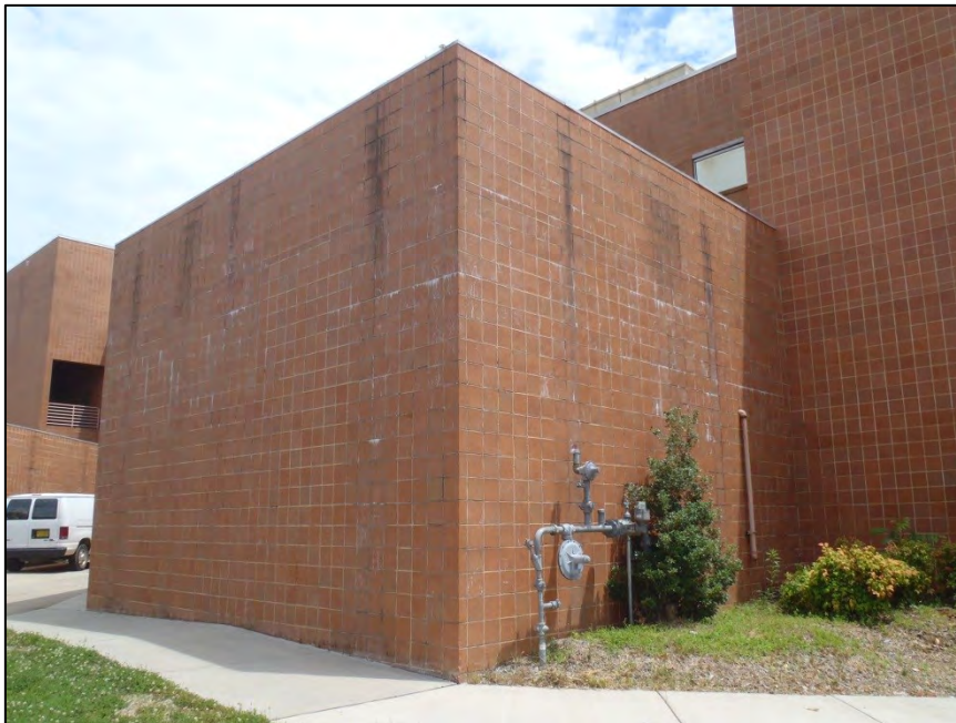
NO. 54 – NORTH ELEVATION AT EXTERIOR SCREEN WALL – EFFLORESCENCE AT EXTERIOR BRICK VENEER
