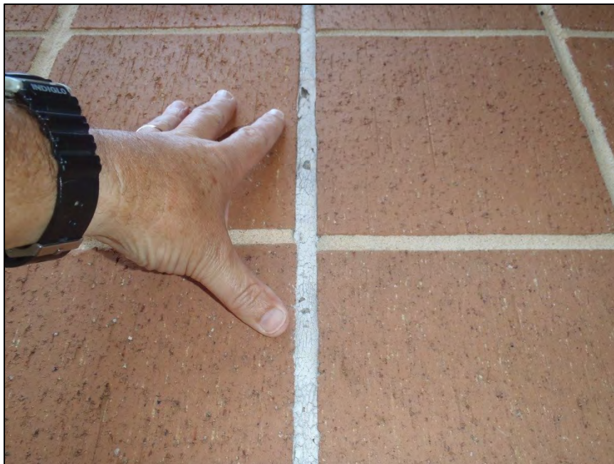
NO. 37 – NORTH ELEVATION – DETERIORATED JOINT SEALANT
