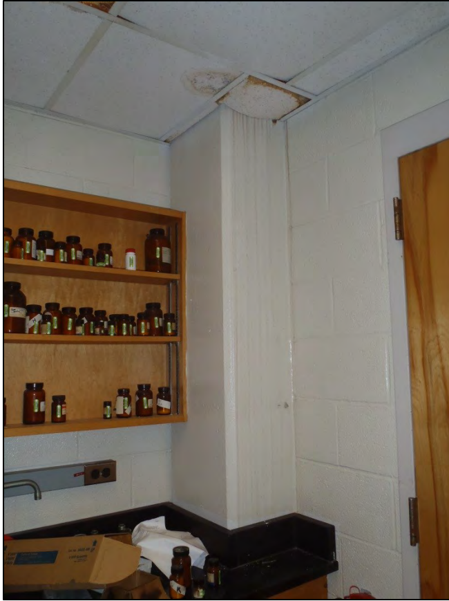
NO. 141 – SECOND FLOOR ROOM 243 – DAMAGED CEILING TILES FROM WATER INFILTRATION
