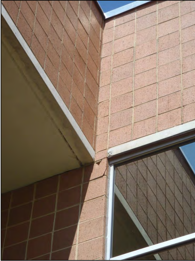
NO. 88 – SOUTHWEST ELEVATION – CRACKED INDIVIDUAL BRICK MASONRY UNITS
