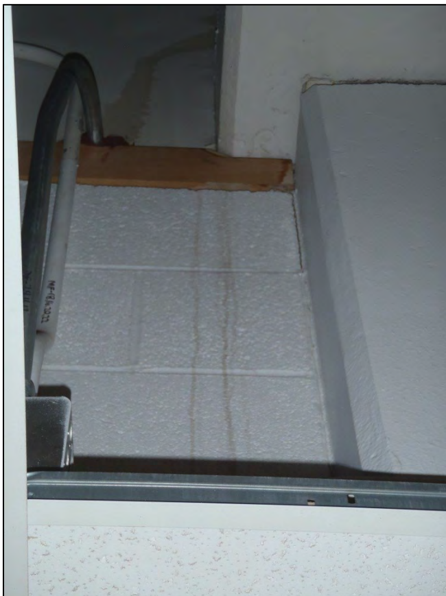
NO. 132 – SECOND FLOOR GENERAL CHEMISTRY LABORATORY 207 – WATER STAINED INTERIOR PARTITION WALL FROM WATER INFILTRATION
