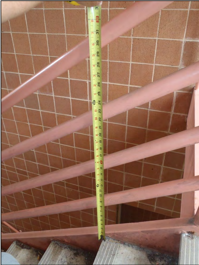
NO. 70 – NORTH ELEVATION AT WEST EXTERIOR STAIRWELL – INADEQUATE GUARDRAIL HEIGHT AT STAIRS
