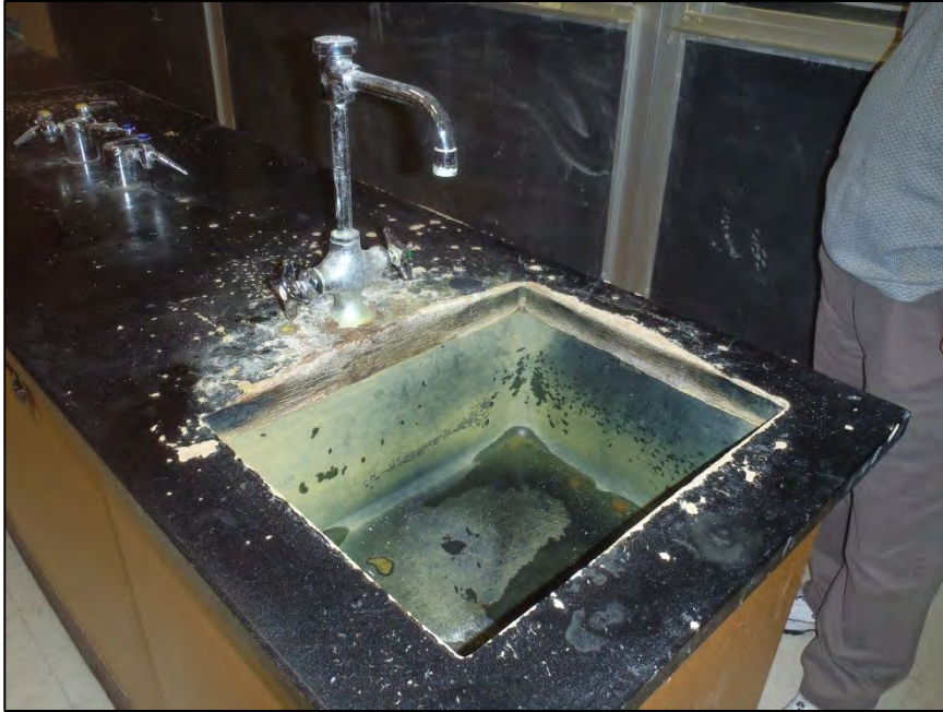
NO. 106 – SOUTHEAST FIRST FLOOR AUDITORIUM – SEVERELY DETERIORATED COUNTERTOP, SINK, AND PLUMBING FIXTURES
