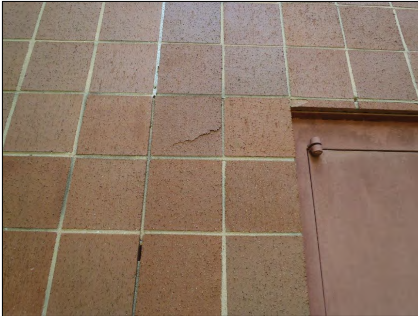
NO. 34 – EAST ELEVATION – CRACKED INDIVIDUAL MASONRY UNIT
