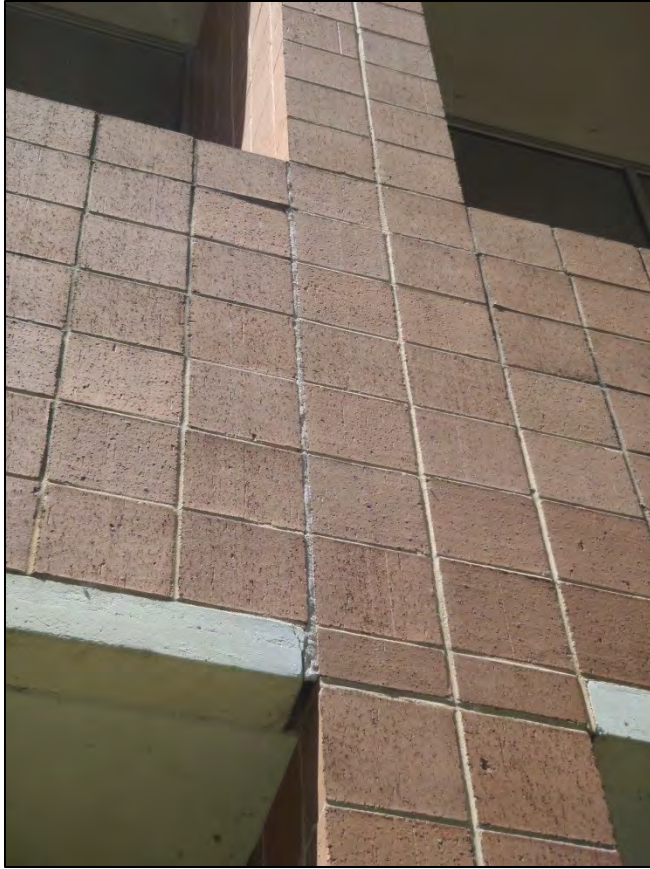
NO. 97 – SOUTH ELEVATION – DETERIORATED JOINT SEALANT
