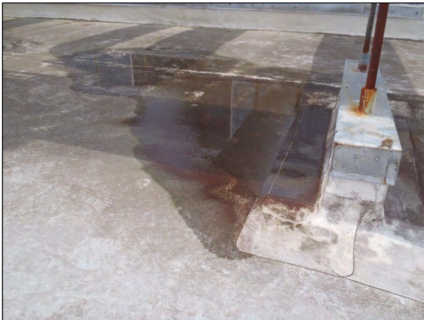
NO. 196 – ROOF – PONDING WATER
