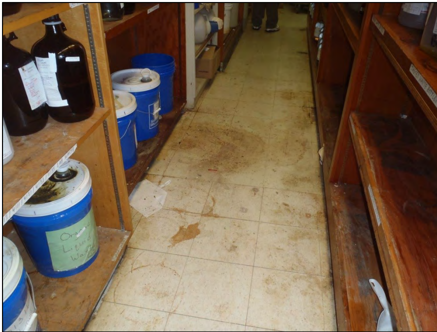
NO. 160 – SECOND FLOOR ROOM 225A – CHEMICALLY STAINED FURNITURE AND FLOOR FINISHES
