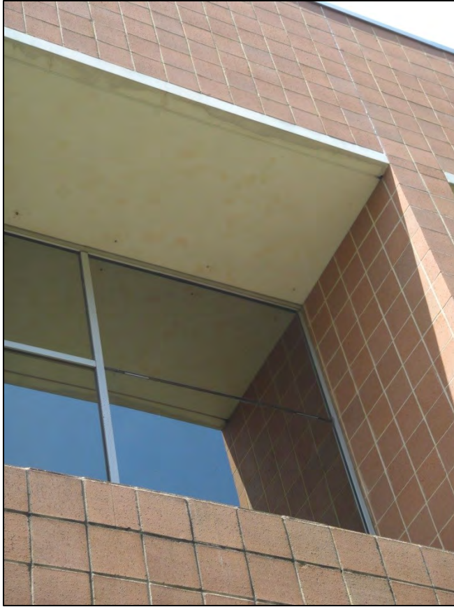
NO. 86 – SOUTH ELEVATION – DISPLACED WINDOW FRAMING
