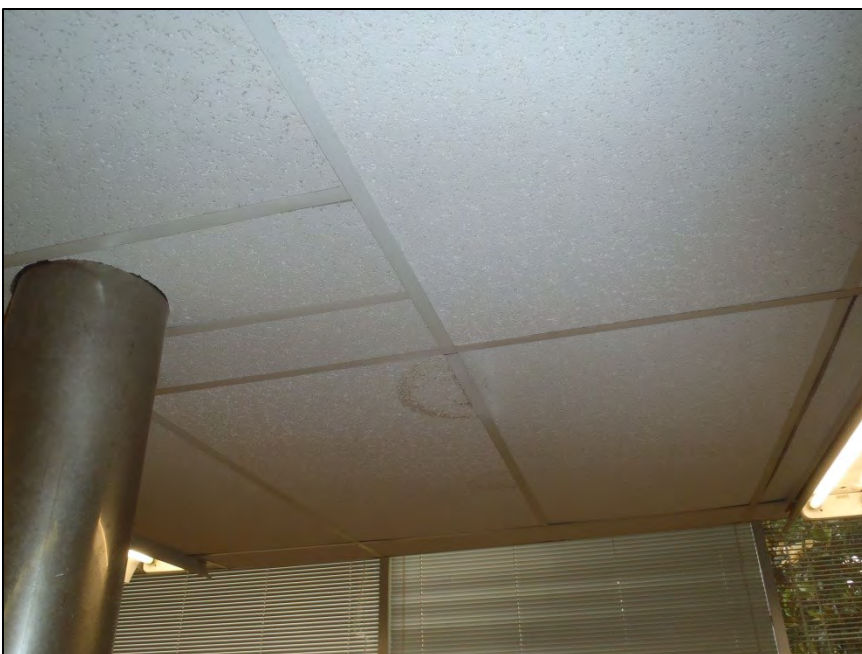
NO. 130 – SECOND FLOOR GENERAL CHEMISTRY LABORATORY 207 – DAMAGED CEILING TILES FROM WATER INFILTRATION
