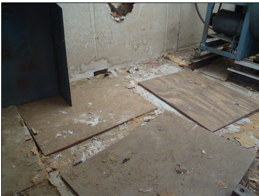
NO. 216 – ROOF SKYLIGHT/MECHANICAL ENCLOSURE – WATER DAMAGED INTERIOR FINISHES
