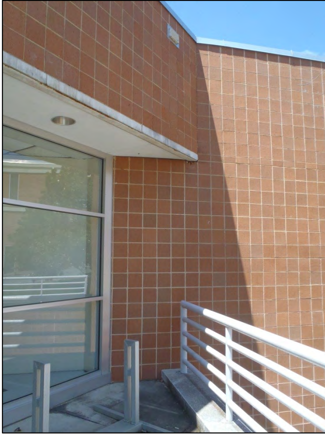
NO. 31 – SOUTHEAST ELEVATION AT MAIN ENTRANCE – CRACKED BRICK VENEER AT GIRDER BEARING
