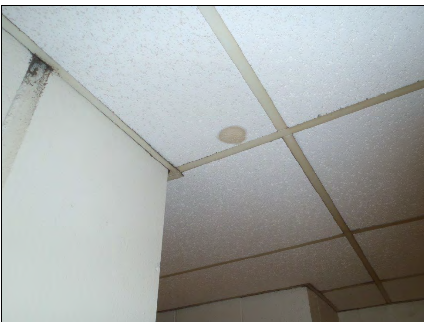
NO. 157 – SECOND FLOOR CORRIDOR – WATER DAMAGED CEILING TILES FROM WATER INFILTRATION
