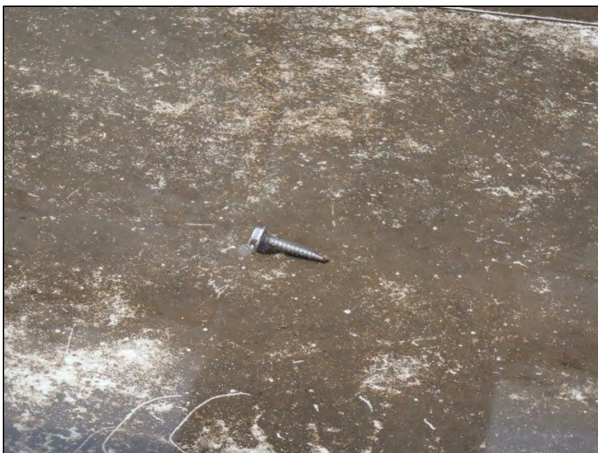
NO. 203 – ROOF – SHARP FOREIGN DEBRIS
