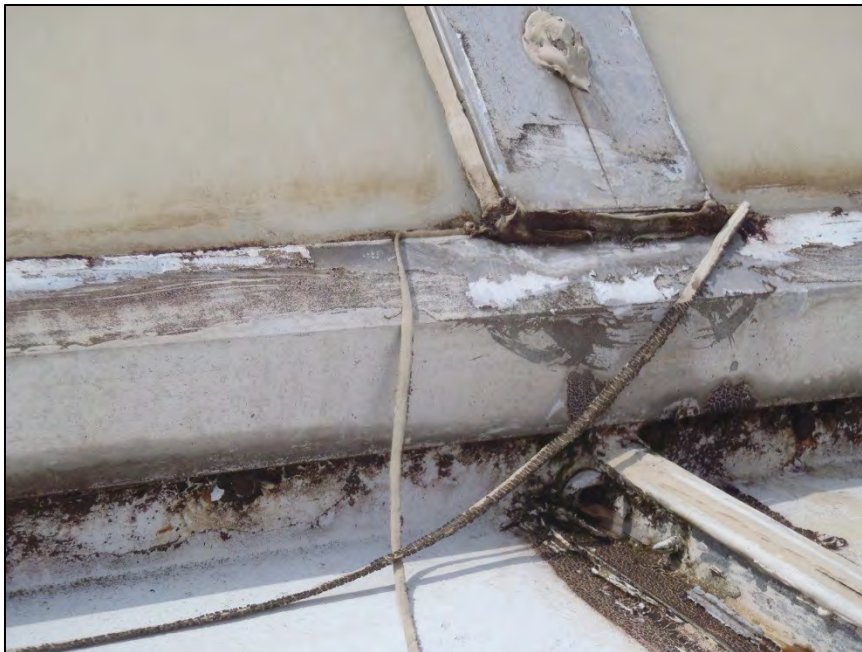
NO. 207 – ROOF SKYLIGHT/MECHANICAL ENCLOSURE – DETERIORATED JOINT SEALANTS ALLOWING WATER INFILTRATION
