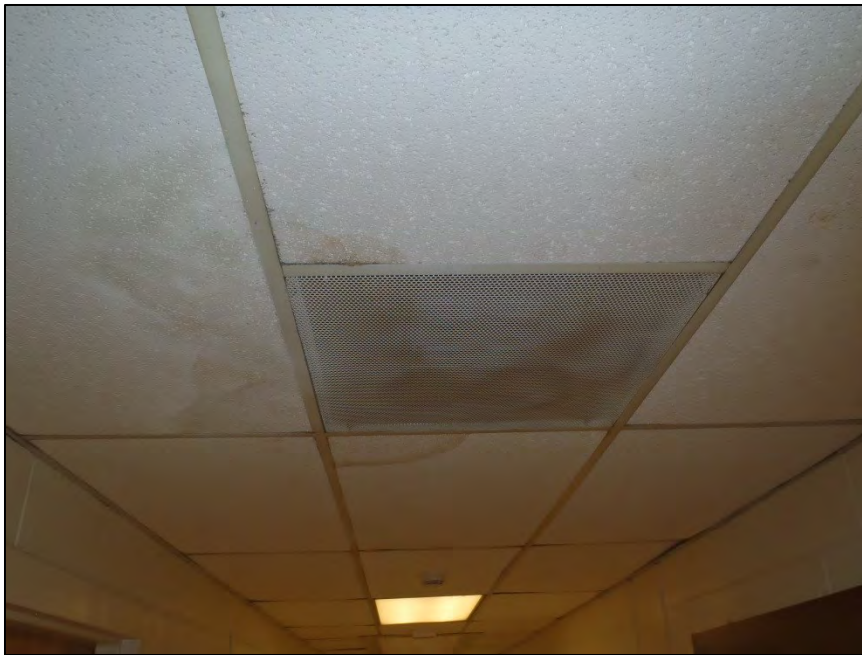
NO. 155 – SECOND FLOOR CORRIDOR – WATER DAMAGED CEILING TILES FROM WATER INFILTRATION
