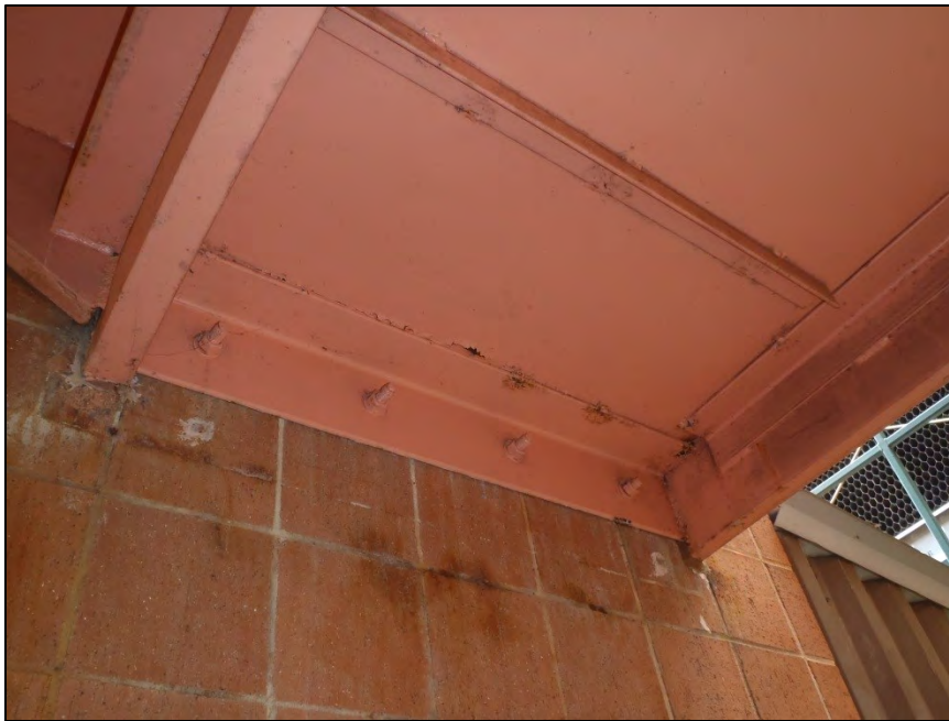
NO. 59 – NORTH ELEVATION AT CENTER EXTERIOR STAIRWELL – DETERIORATED LANDING FRAMING
