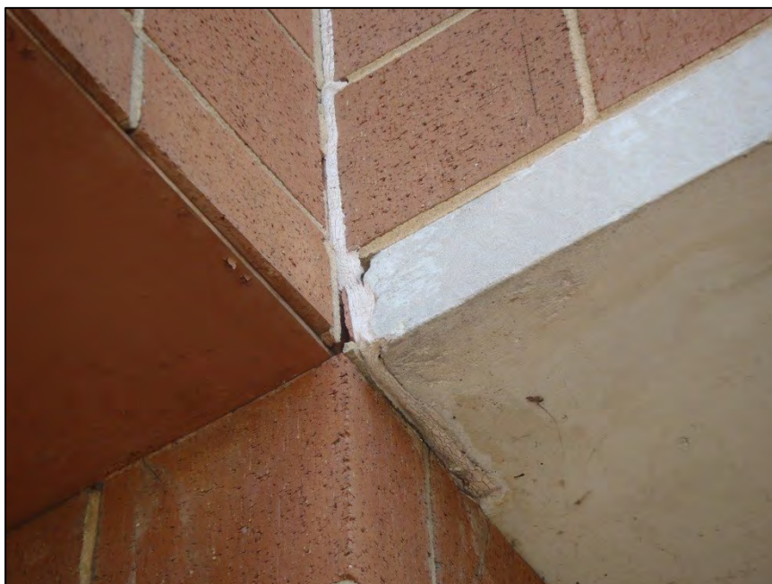
NO. 38 – NORTH ELEVATION – DETERIORATED JOINT SEALANT
