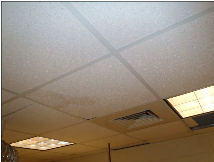
NO. 149 – SECOND FLOOR ROOM 274 RESEARCH LABORATORY – DAMAGED CEILING TILES FROM WATER INFILTRATION
