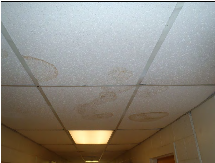
NO. 144 – SECOND FLOOR CORRIDOR – DAMAGED CEILING TILES FROM WATER INFILTRATION
