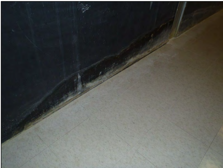
NO. 104 – SOUTHEAST FIRST FLOOR AUDITORIUM – WATER INFILTRATION AT BASE OF WALL
