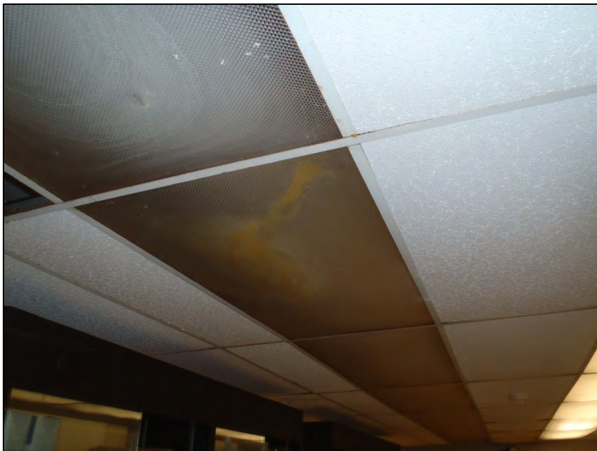
NO. 139 – SECOND FLOOR ROOM 243 – STAINED LIGHT FIXTURE DUE TO WATER INFILTRATION
