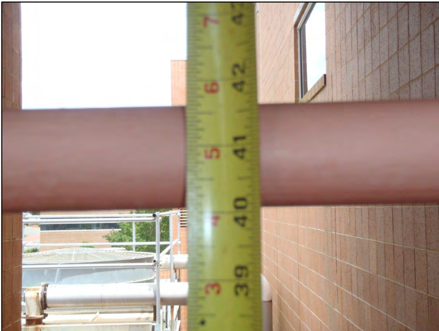
NO. 66 – NORTH ELEVATION AT CENTER EXTERIOR STAIRWELL – INADEQUATE GUARDRAIL HEIGHT
