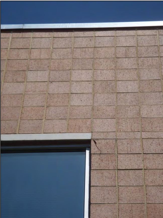
NO. 91 – SOUTHWEST ELEVATION – CRACKED INDIVIDUAL BRICK MASONRY UNITS
