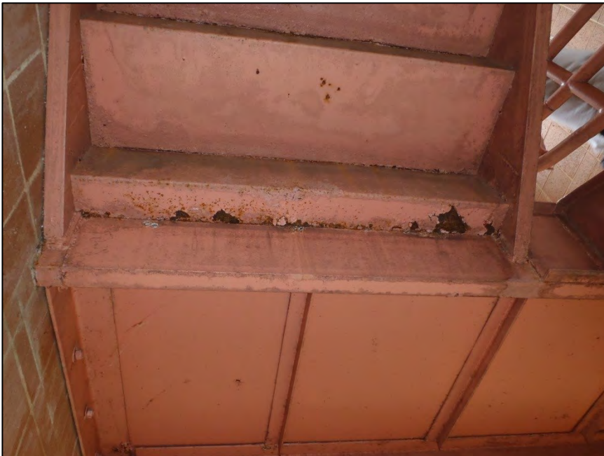
NO. 72 – NORTH ELEVATION AT WEST EXTERIOR STAIRWELL – DETERIORATED STAIR FRAMING
