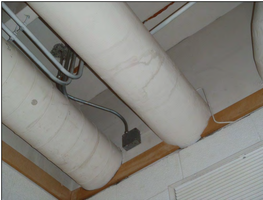
NO. 159 – SECOND FLOOR ROOM 221 – WATER STAINED DUCT WORK FROM WATER INFILTRATION AND/OR CONDENSATION
