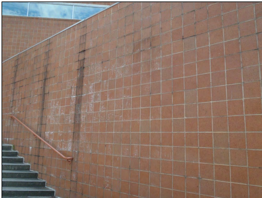
NO. 47 – NORTH ELEVATION AT EXTERIOR SCREEN WALL – EFFLORESCENCE AT EXTERIOR BRICK VENEER
