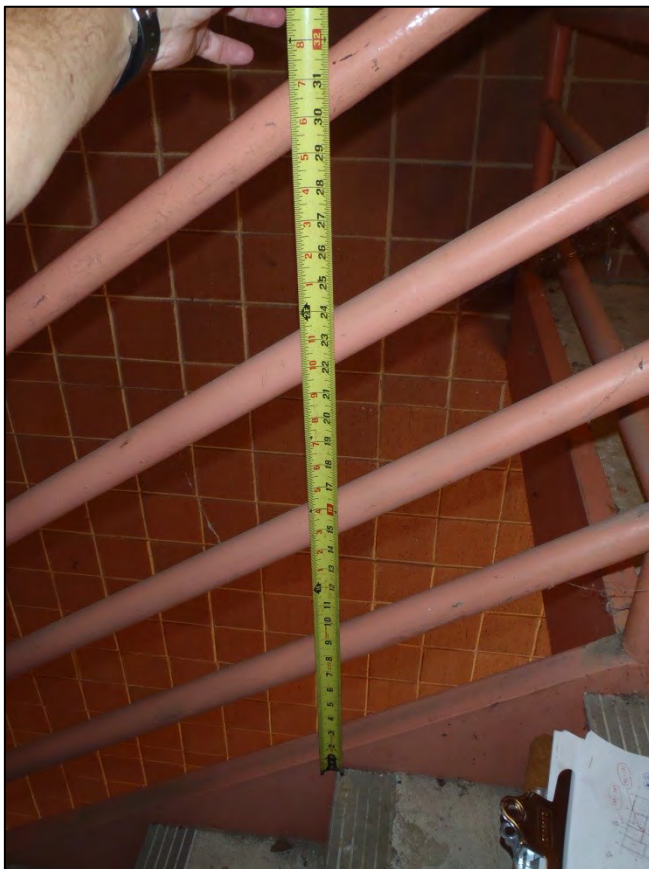
NO. 40 – NORTH ELEVATION AT EAST EXTERIOR STAIRWELL – INADEQUATE GUARDRAIL HEIGHT AT STAIRS
