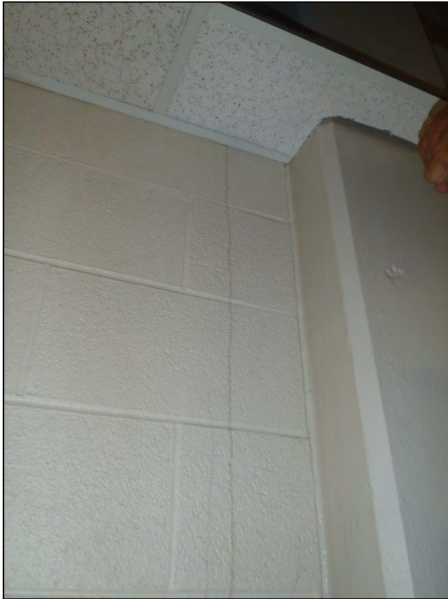
NO. 131 – SECOND FLOOR GENERAL CHEMISTRY LABORATORY 207 – WATER STAINED INTERIOR PARTITION WALL FROM WATER INFILTRATION
