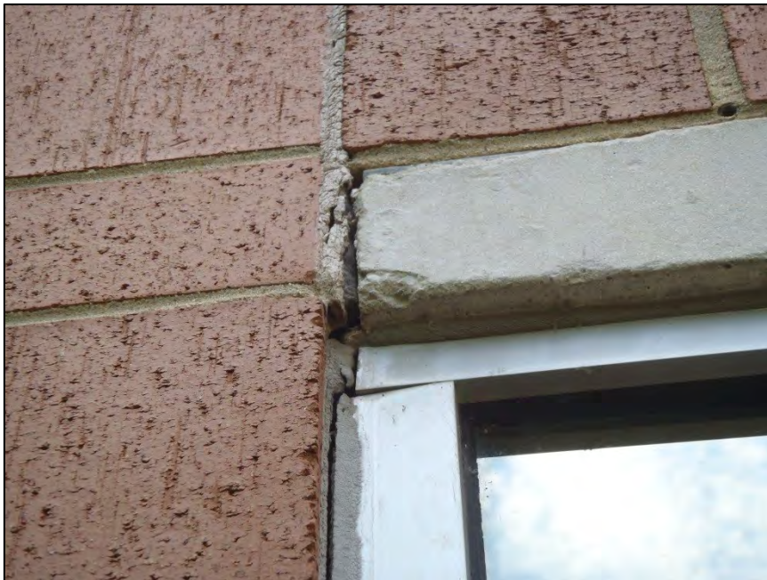
NO. 36 – NORTH ELEVATION – DETERIORATED EXTERIOR JOINT REQUIRING JOINT SEALANT
