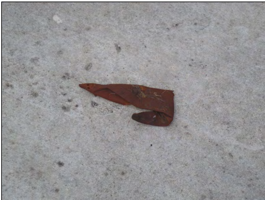
NO. 202 – ROOF – SHARP FOREIGN DEBRIS
