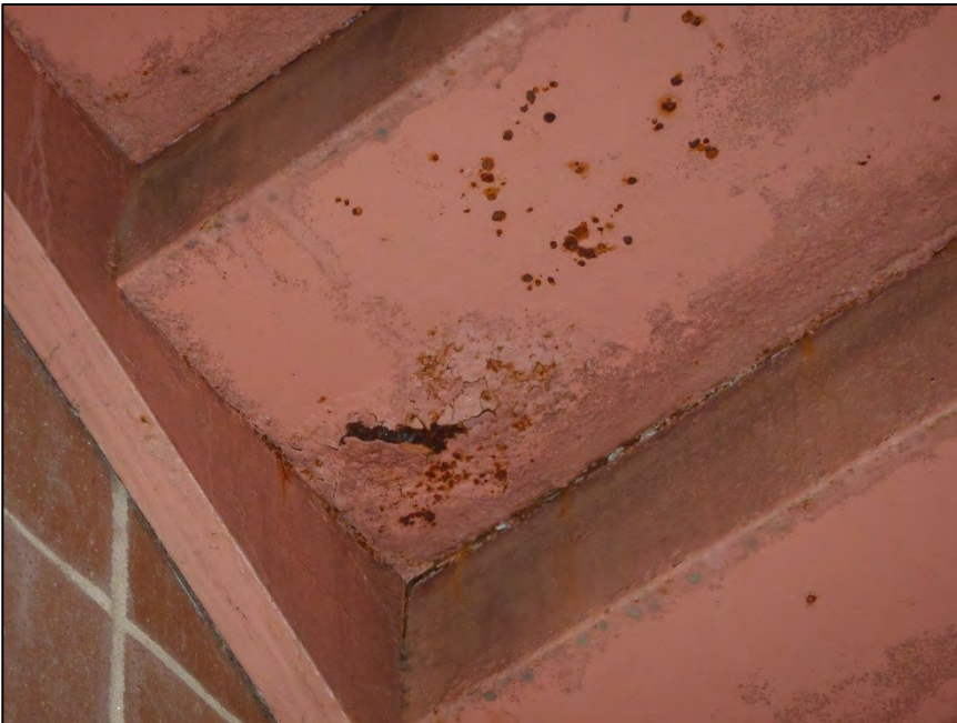
NO. 74 – NORTH ELEVATION AT WEST EXTERIOR STAIRWELL – DETERIORATED STAIR FRAMING
