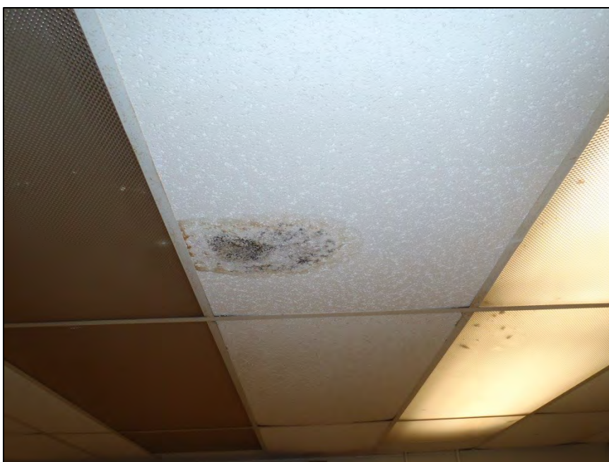
NO. 140 – SECOND FLOOR ROOM 243 – DAMAGED CEILING TILES FROM WATER INFILTRATION
