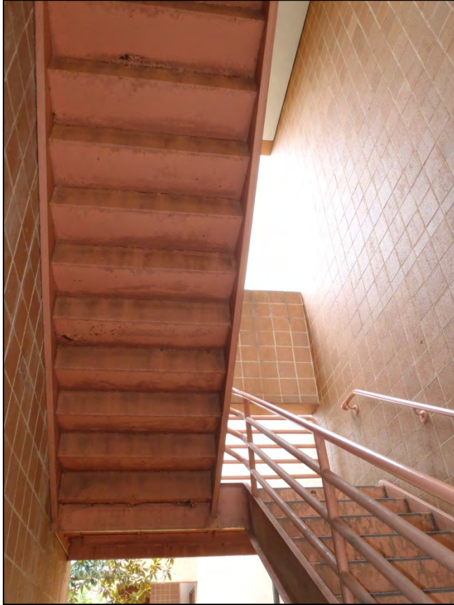
NO. 71 – NORTH ELEVATION AT WEST EXTERIOR STAIRWELL – DETERIORATED STAIR FRAMING
