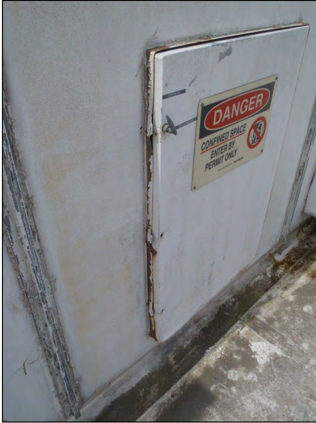
NO. 210 – ROOF SKYLIGHT/MECHANICAL ENCLOSURE – TYPICAL CONFINED SPACE ACCESS
