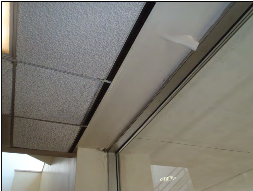
NO. 100 – FIRST FLOOR AT SOUTHEAST ENTRY PLAZA – WATER INFILTRATION
