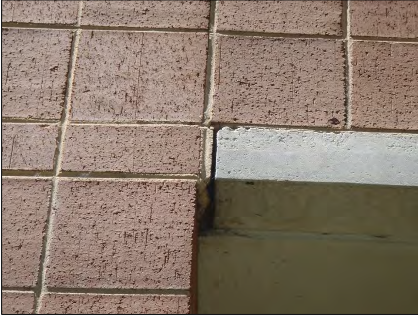
NO. 95 – SOUTH ELEVATION – DETERIORATED JOINT REQUIRING JOINT SEALANT
