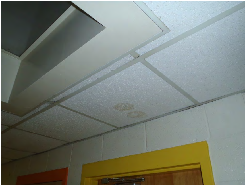
NO. 125 – SECOND FLOOR CORRIDOR – DAMAGED CEILING TILE FROM WATER INFILTRATION
