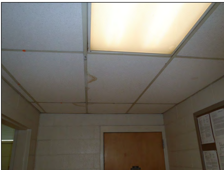
NO. 145 – SECOND FLOOR CORRIDOR – DAMAGED CEILING TILES FROM WATER INFILTRATION
