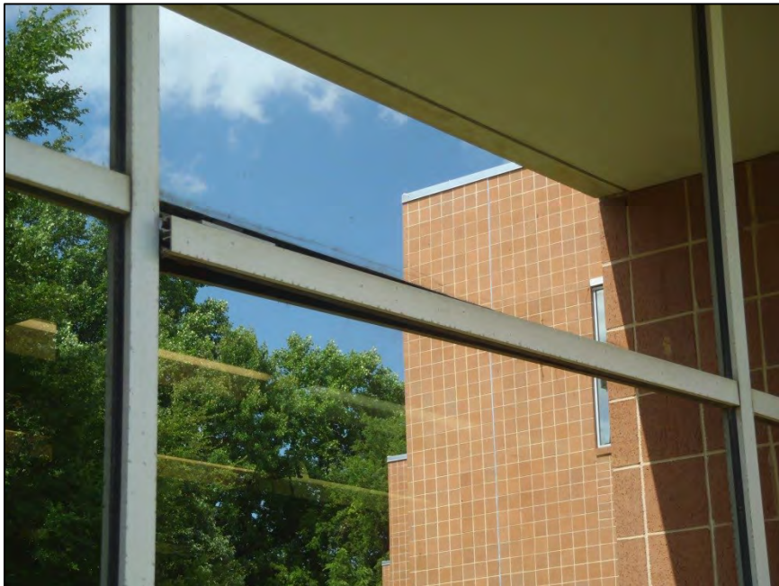
NO. 87 – SOUTH ELEVATION – DISPLACED WINDOW FRAMING
