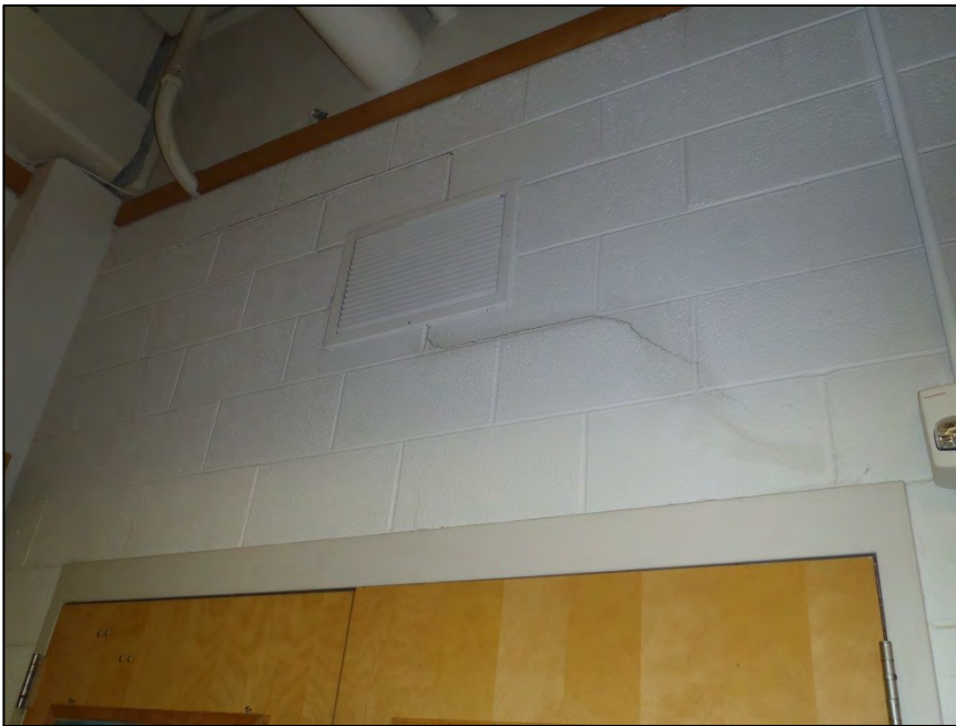
NO. 114 – FIRST FLOOR – INTERIOR CRACKS IN A CONCRETE MASONRY PARTITION WALL
