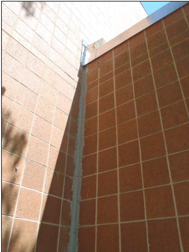
NO. 79 – WEST ELEVATION AT BASEMENT ADDITION – DETERIORATED JOINT SEALANT
