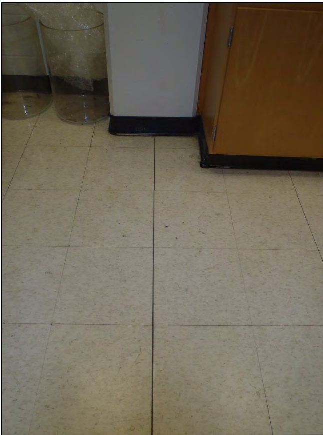
NO. 118 – FIRST FLOOR – DISPLACED INTERIOR FLOOR FINISHES
