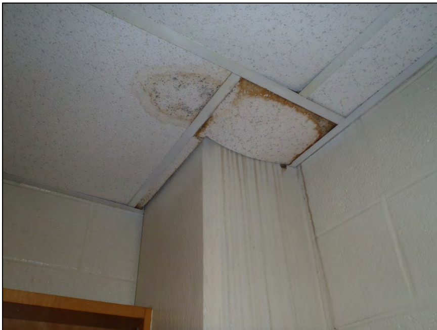
NO. 142 – SECOND FLOOR ROOM 243 – DAMAGED CEILING TILES FROM WATER INFILTRATION
