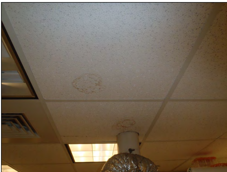
NO. 148 – SECOND FLOOR ROOM 274 RESEARCH LABORATORY – DAMAGED CEILING TILES FROM WATER INFILTRATION
