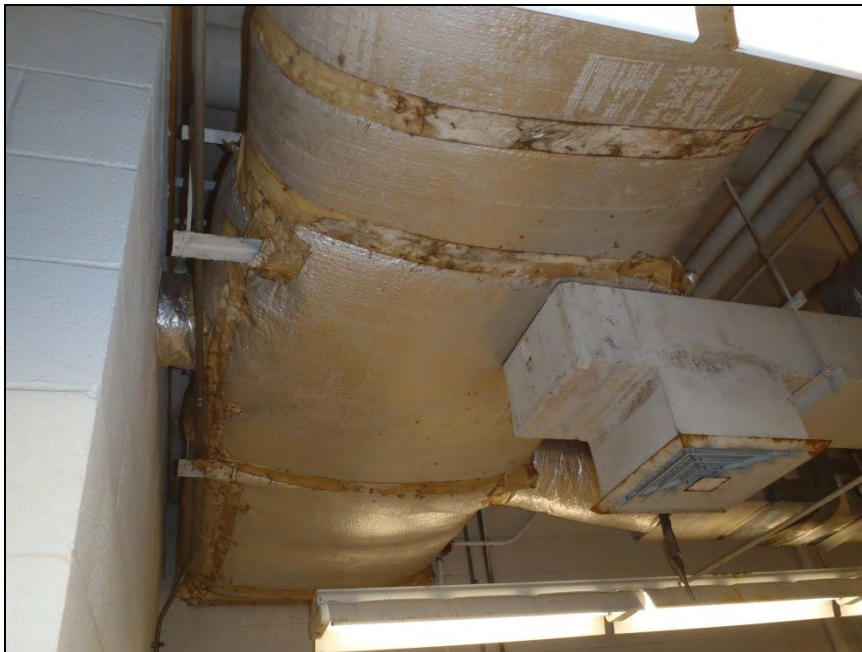
NO. 138 – SECOND FLOOR ROOM 241 – WATER STAINED DUCT WORK FROM WATER INFILTRATION AND/OR CONDENSATION
