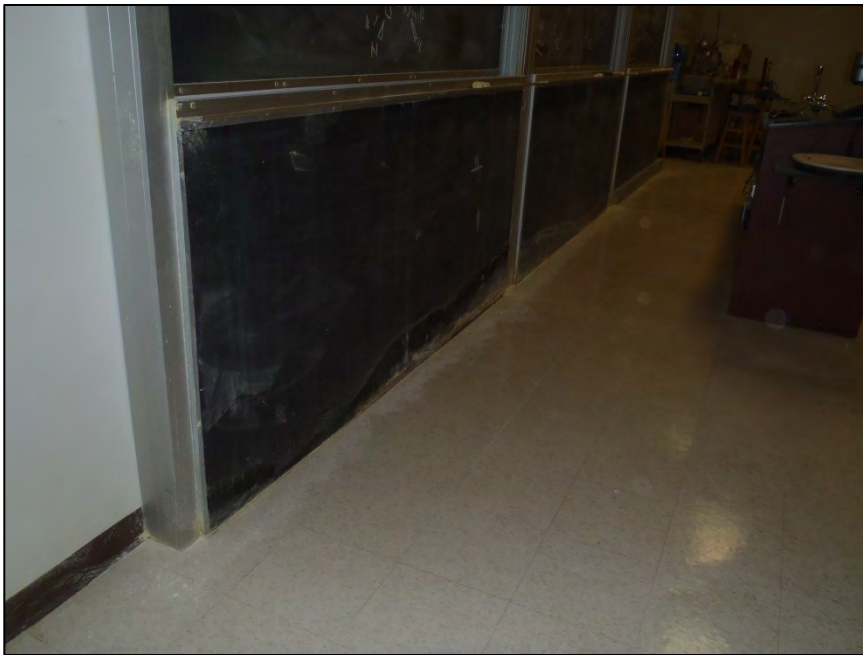
NO. 103 – SOUTHEAST FIRST FLOOR AUDITORIUM – WATER INFILTRATION AT BASE OF WALL
