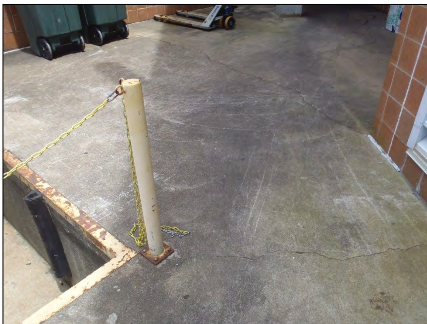
NO. 50 – NORTH ELEVATION AT LOADING DOCK – DETERIORATED EXTERIOR CONCRETE SLAB
