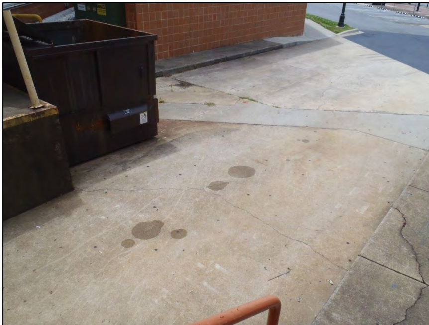
NO. 49 – NORTH ELEVATION AT LOADING DOCK – DETERIORATED EXTERIOR CONCRETE SLAB
