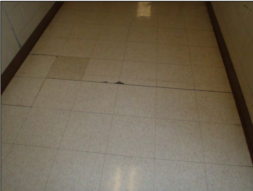
NO. 109 – FIRST FLOOR INTERIOR HALLWAY – CRACKED FLOOR FINISHES
