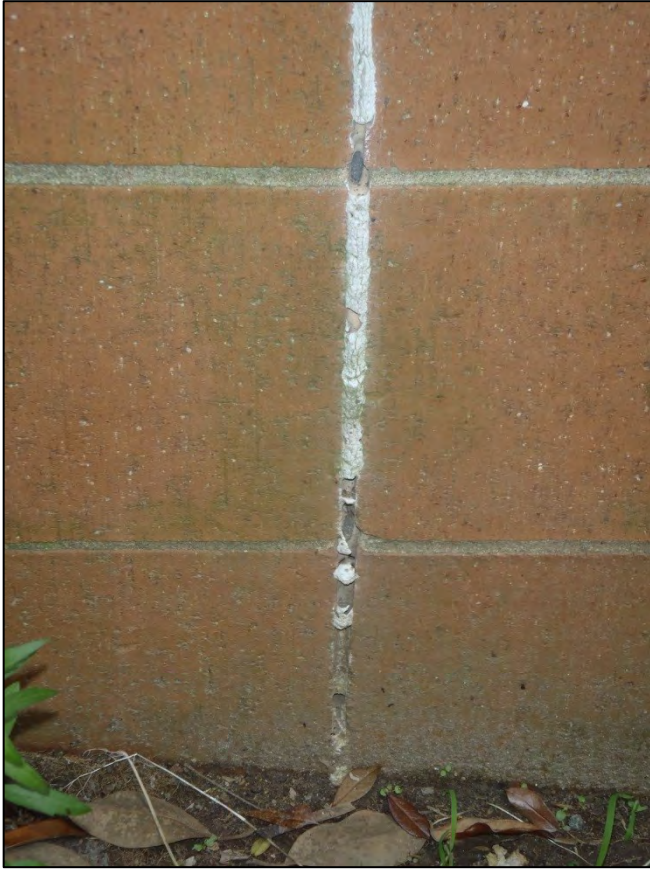
NO. 33 – EAST ELEVATION – DETERIORATED JOINT SEALANT
