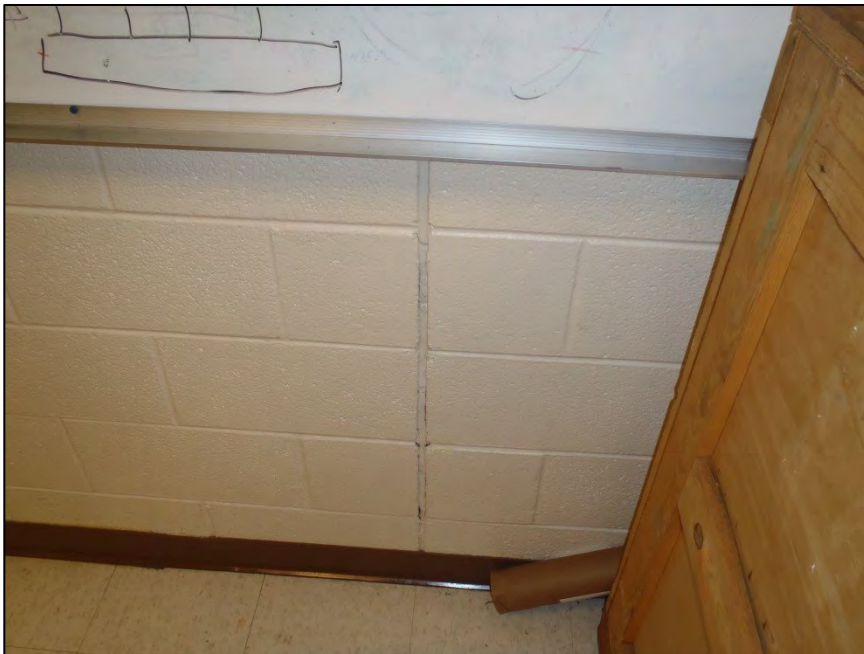
NO. 107 – FIRST FLOOR RESEARCH LABORATORY – DETERIORATED INTERIOR JOINT SEALANT
