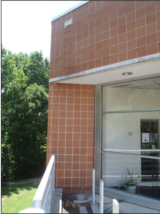
NO. 29 – SOUTHEAST ELEVATION AT MAIN ENTRANCE – DISPLACED BRICK VENEER AT GIRDER BEARING
