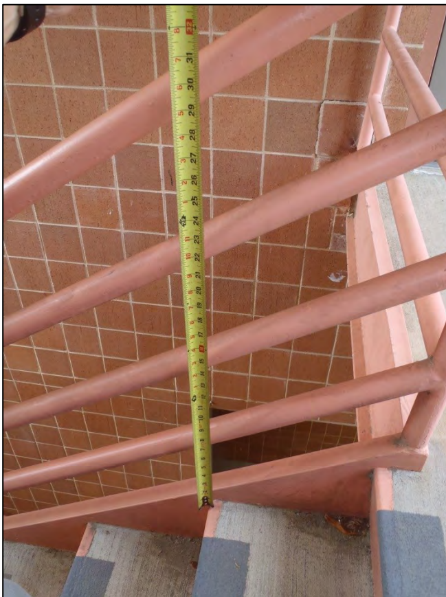
NO. 58 – NORTH ELEVATION AT CENTER EXTERIOR STAIRWELL – INADEQUATE GUARDRAIL HEIGHT AT STAIRS
