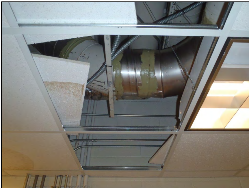
NO. 147 – SECOND FLOOR ROOM 274 RESEARCH LABORATORY – DAMAGED CEILING TILES FROM WATER INFILTRATION
