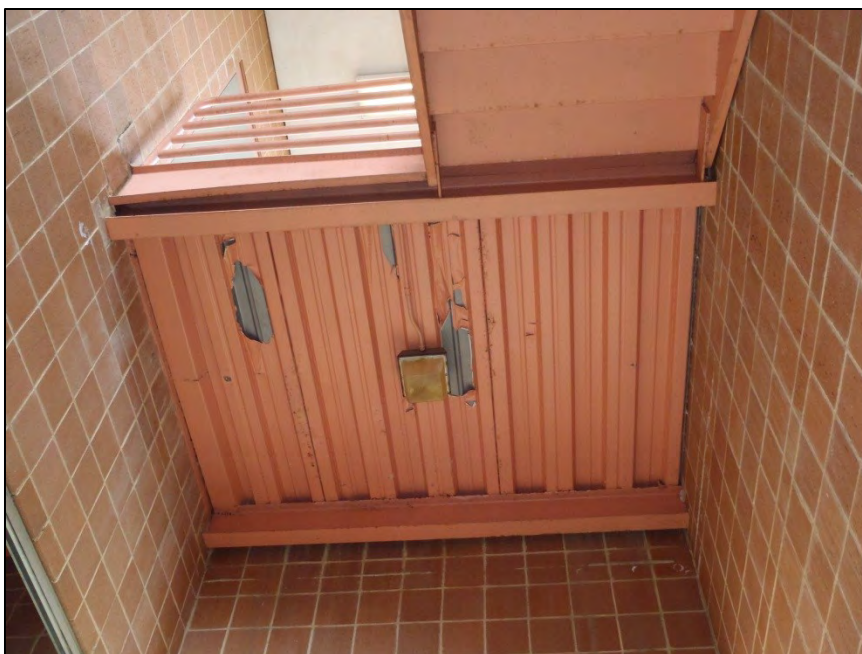
NO. 61 – NORTH ELEVATION AT CENTER EXTERIOR STAIRWELL – DETERIORATED LANDING FRAMING
