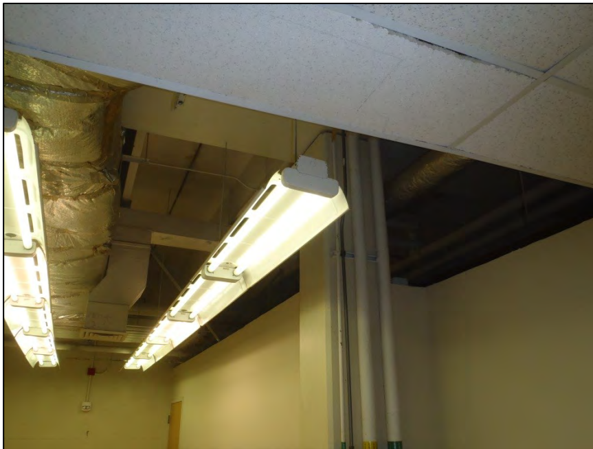
NO. 134 – SECOND FLOOR GENERAL CHEMISTRY LABORATORY 207 – MISSING CEILING TILES
