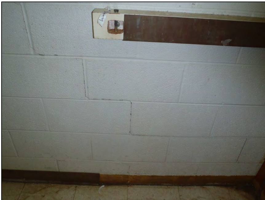
NO. 164 – SECOND FLOOR ROOM 225 – CRACKED INTERIOR CONCRETE MASONRY WALL
