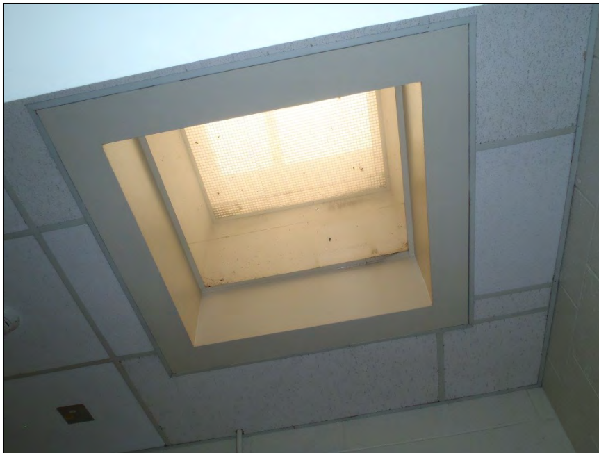
NO. 135 – SECOND FLOOR CORRIDOR – DAMAGED CEILING TILES FROM WATER INFILTRATION
