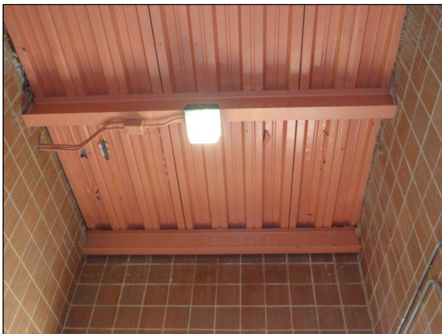
NO. 43 – NORTH ELEVATION AT EAST EXTERIOR STAIRWELL – DETERIORATED LANDING FRAMING
