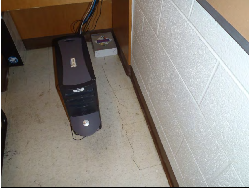
NO. 117 – FIRST FLOOR – CRACKED INTERIOR FLOOR FINISHES
