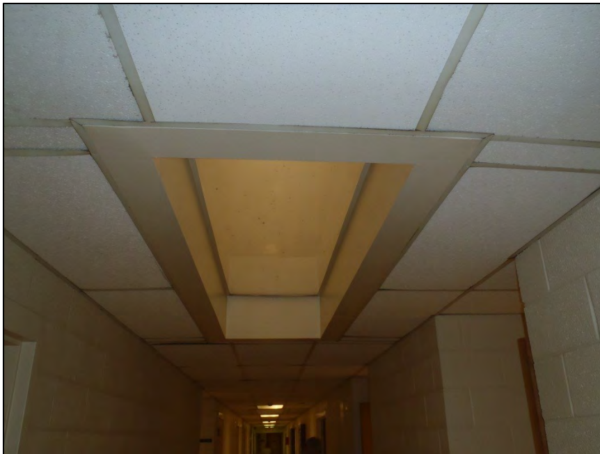
NO. 152 – SECOND FLOOR CORRIDOR – WATER STAINED SKYLIGHT DUE TO WATER INFILTRATION
