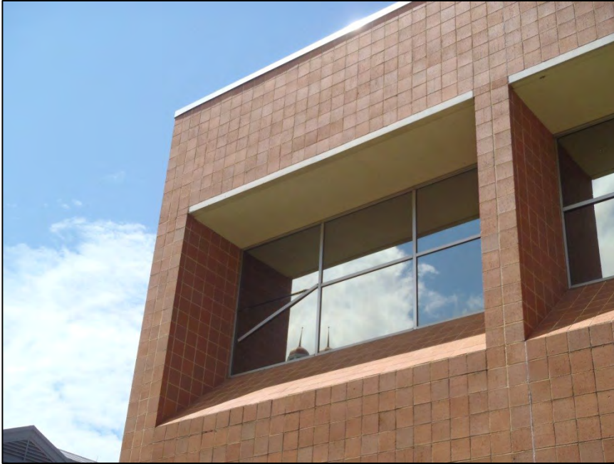
NO. 84 – SOUTH ELEVATION – DISPLACED WINDOW FRAMING
