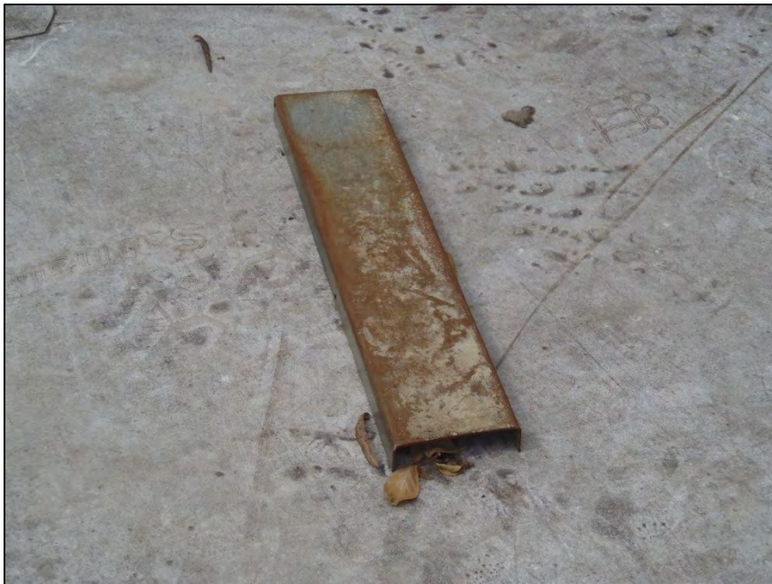
NO. 201 – ROOF – SHARP FOREIGN DEBRIS
