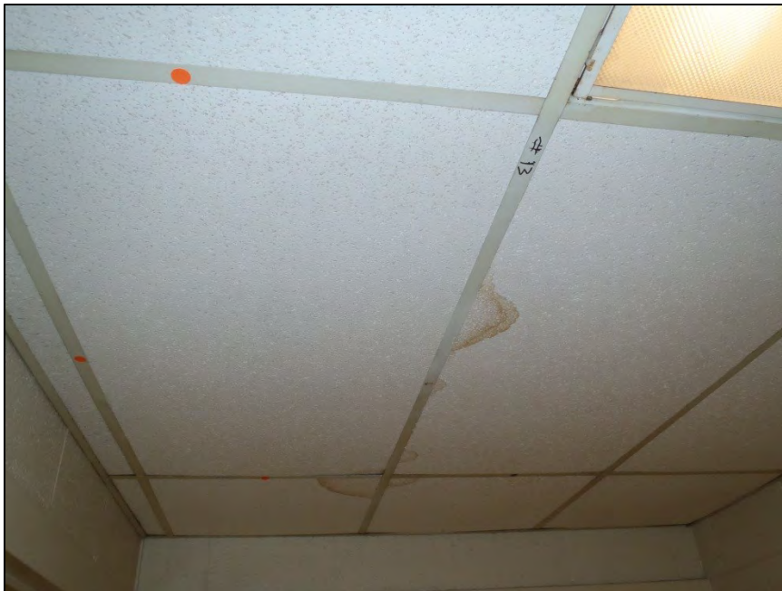
NO. 146 – SECOND FLOOR CORRIDOR – DAMAGED CEILING TILES FROM WATER INFILTRATION
