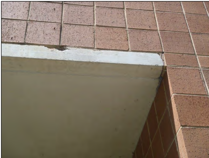
NO. 98 – SOUTH ELEVATION – CONCRETE SPALL AND DETERIORATED JOINT REQUIRING JOINT SEALANT
