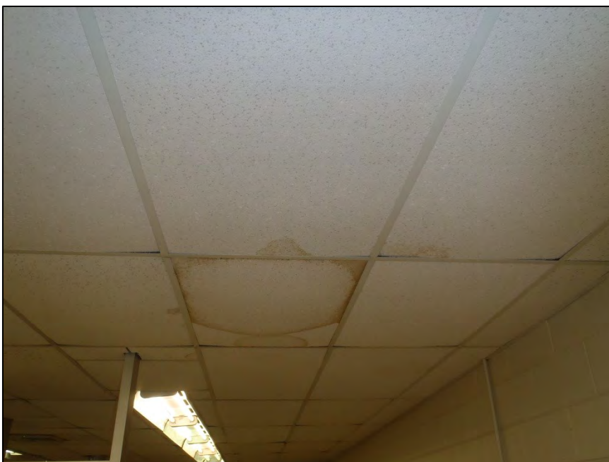
NO. 127 – SECOND FLOOR GENERAL CHEMISTRY LABORATORY 207 – DAMAGED CEILING TILES FROM WATER INFILTRATION
