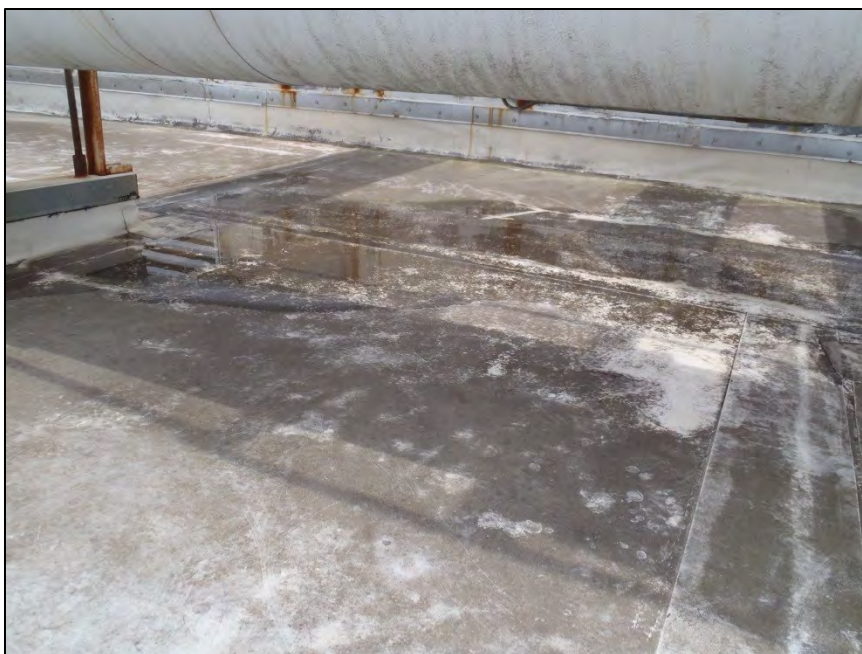
NO. 197 – ROOF – PONDING WATER
