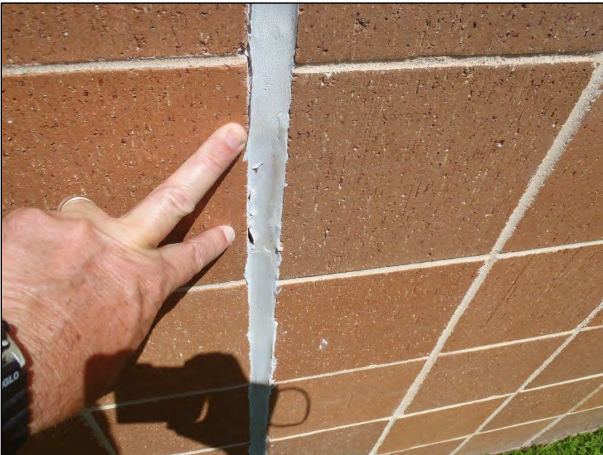
NO. 93 – SOUTHWEST ELEVATION – DETERIORATED JOINT SEALANT
