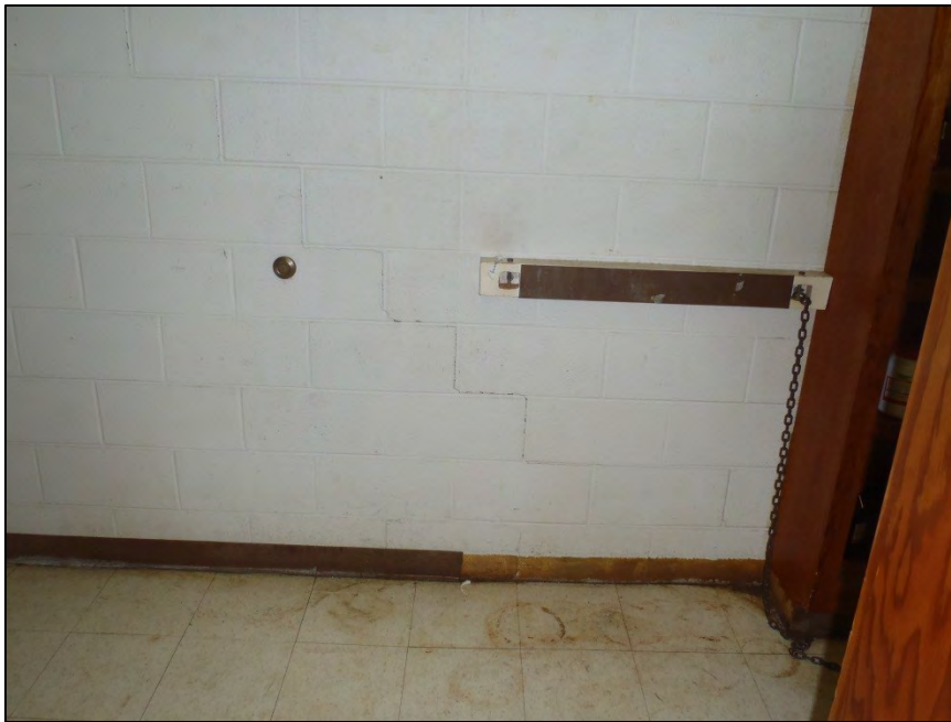
NO. 163 – SECOND FLOOR ROOM 225 – CRACKED INTERIOR CONCRETE MASONRY WALL
