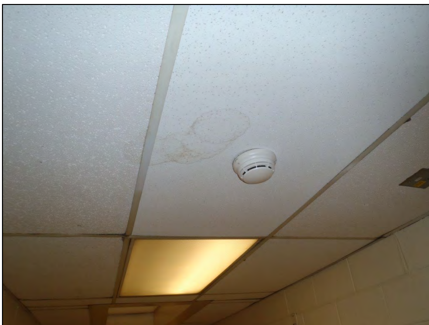
NO. 154 – SECOND FLOOR CORRIDOR – WATER DAMAGED CEILING TILES FROM WATER INFILTRATION
