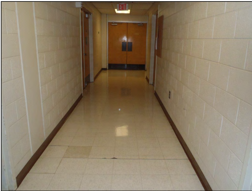
NO. 108 – FIRST FLOOR INTERIOR HALLWAY – CRACKED FLOOR FINISHES
