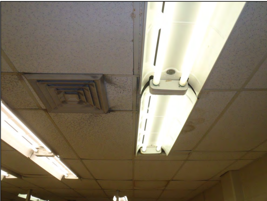
NO. 126 – SECOND FLOOR GENERAL CHEMISTRY LABORATORY 207 – DAMAGED CEILING TILES FROM WATER INFILTRATION
