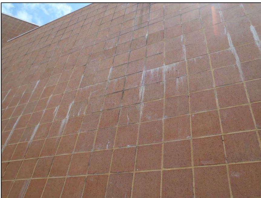
NO. 53 – NORTH ELEVATION AT EXTERIOR SCREEN WALL – EFFLORESCENCE AT EXTERIOR BRICK VENEER
