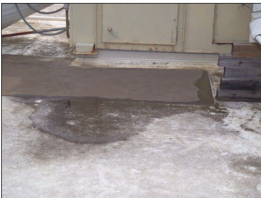
NO. 200 – ROOF – PONDING WATER
