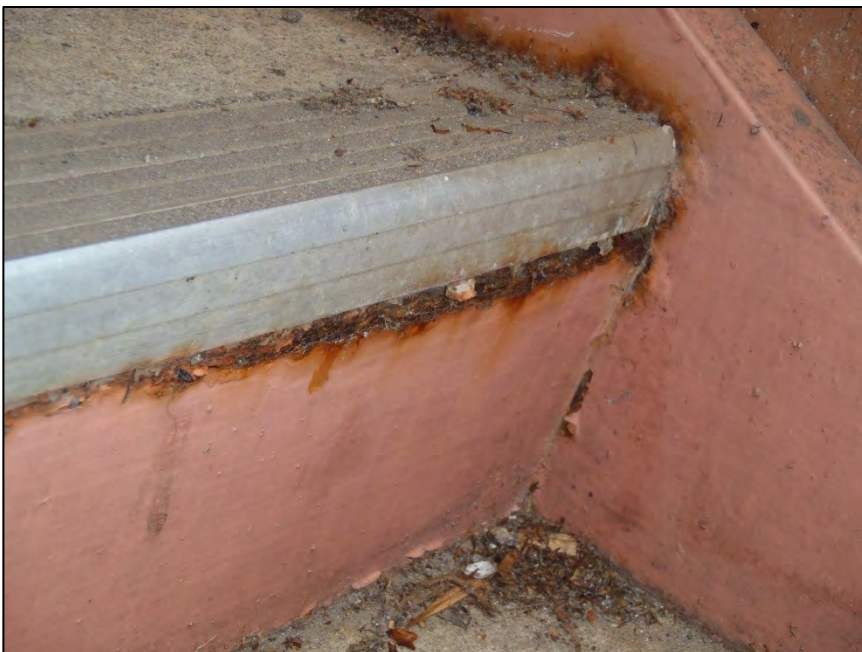
NO. 75 – NORTH ELEVATION AT WEST EXTERIOR STAIRWELL – DETERIORATED STAIR FRAMING
