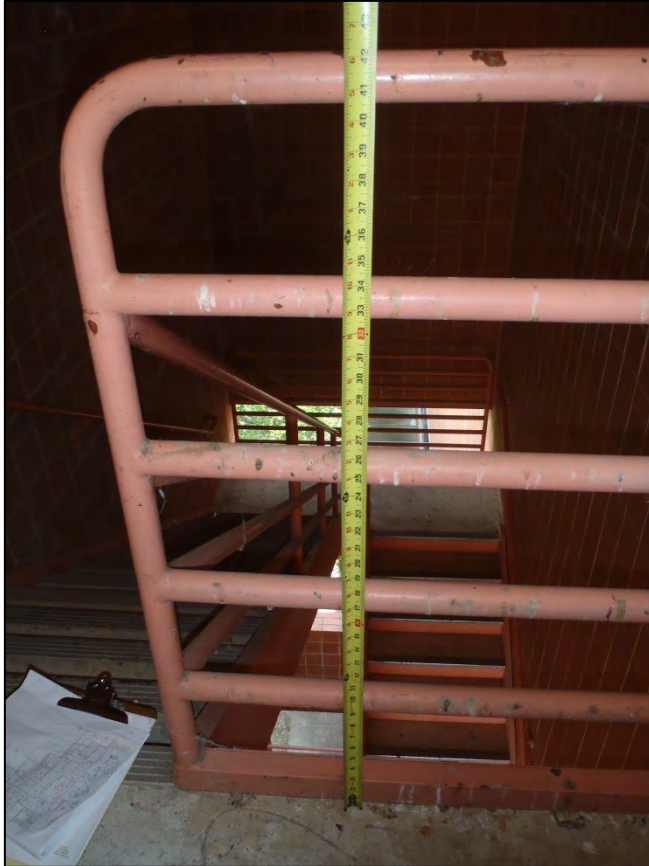
NO. 44 – NORTH ELEVATION AT EAST EXTERIOR STAIRWELL – INADEQUATE GUARDRAIL PICKET SPACINGS
