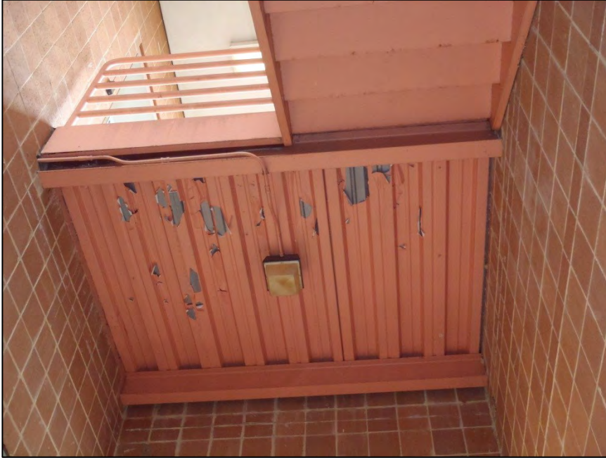
NO. 76 – NORTH ELEVATION AT WEST EXTERIOR STAIRWELL – DETERIORATED LANDING FRAMING
