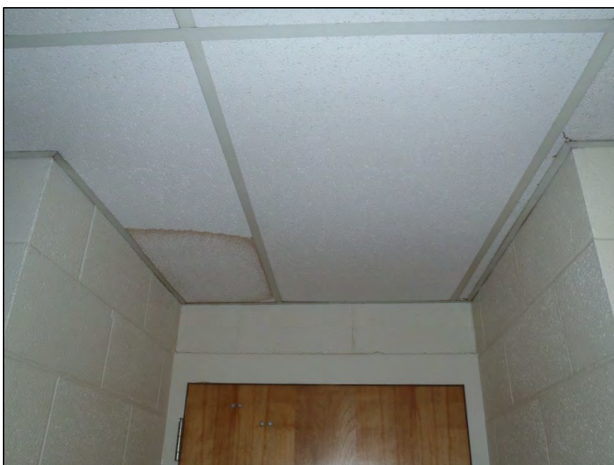
NO. 151 – SECOND FLOOR CORRIDOR – DAMAGED CEILING TILES FROM WATER INFILTRATION
