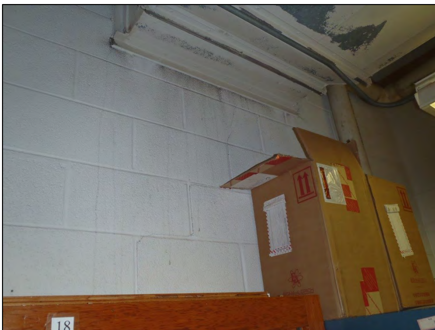
NO. 165 – SECOND FLOOR ROOM 225 – CRACKED INTERIOR CONCRETE MASONRY WALL
