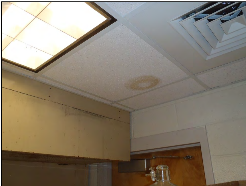
NO. 150 – SECOND FLOOR ROOM 274 RESEARCH LABORATORY – DAMAGED CEILING TILES FROM WATER INFILTRATION
