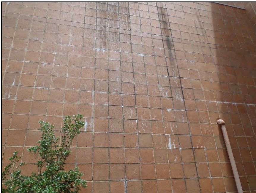
NO. 55 – NORTH ELEVATION AT EXTERIOR SCREEN WALL – EFFLORESCENCE AT EXTERIOR BRICK VENEER
