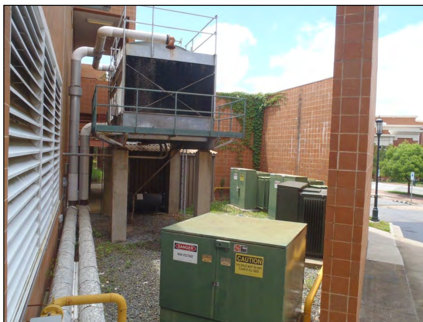
NO. 56 – NORTH ELEVATION AT EXTERIOR SCREEN WALL – EFFLORESCENCE AT EXTERIOR BRICK VENEER
