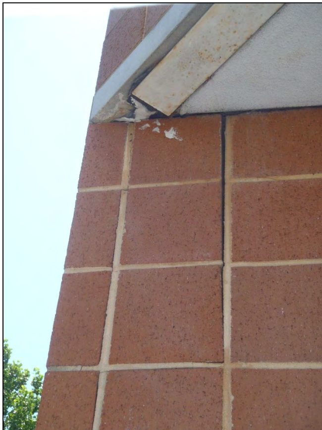
NO. 30 – SOUTHEAST ELEVATION AT MAIN ENTRANCE – DISPLACED BRICK VENEER AT GIRDER BEARING
