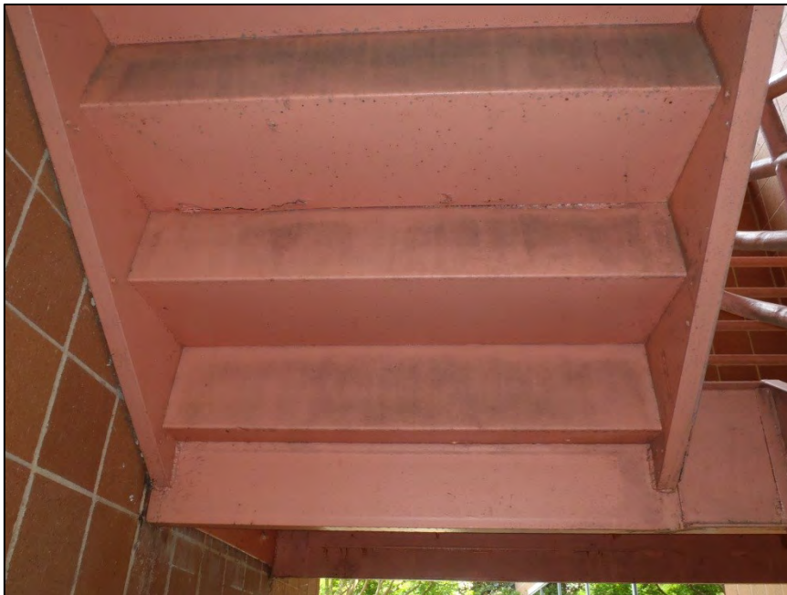
NO. 41 – NORTH ELEVATION AT EAST EXTERIOR STAIRWELL – DETERIORATED STAIR FRAMING
