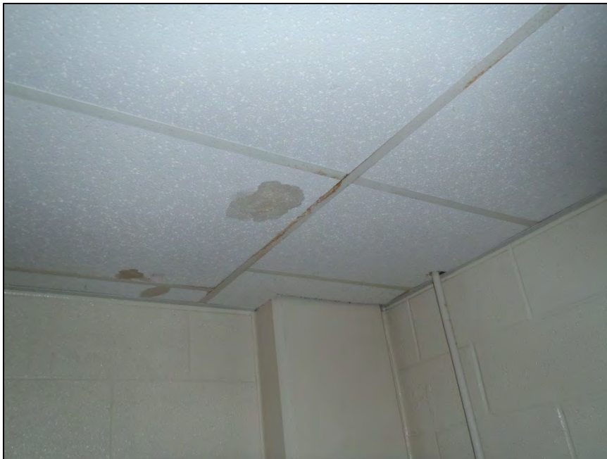
NO. 143 – SECOND FLOOR ROOM 243 – DAMAGED CEILING TILES FROM WATER INFILTRATION
