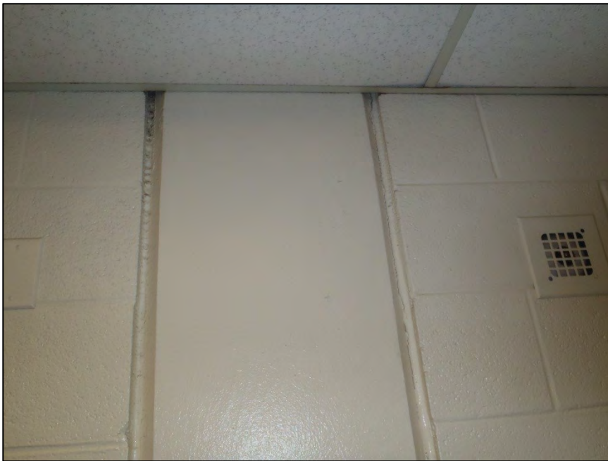
NO. 111 – FIRST FLOOR INTERIOR HALLWAY – DETERIORATED INTERIOR JOINT SEALANTS
