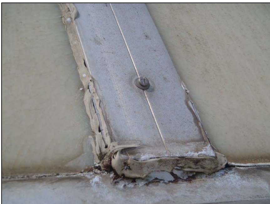
NO. 206 – ROOF SKYLIGHT/MECHANICAL ENCLOSURE – DETERIORATED JOINT SEALANTS ALLOWING WATER INFILTRATION
