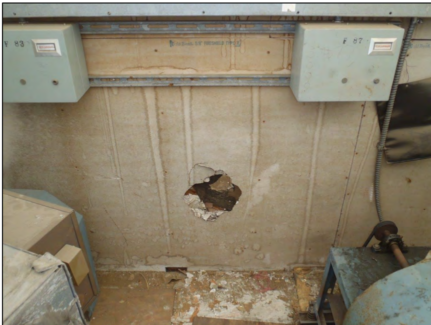
NO. 213 – ROOF SKYLIGHT/MECHANICAL ENCLOSURE – WATER DAMAGED INTERIOR FINISHES
