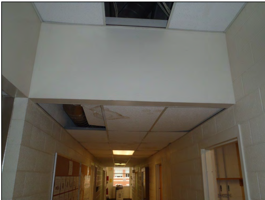
NO. 136 – SECOND FLOOR CORRIDOR – DAMAGED CEILING TILES FROM WATER INFILTRATION
