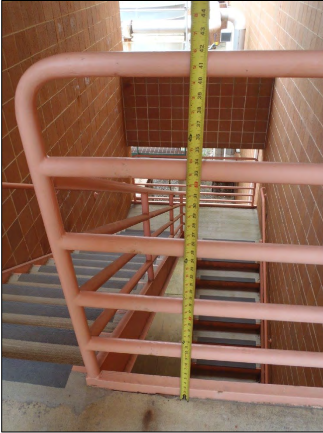
NO. 65 – NORTH ELEVATION AT CENTER EXTERIOR STAIRWELL – INADEQUATE GUARDRAIL HEIGHT
