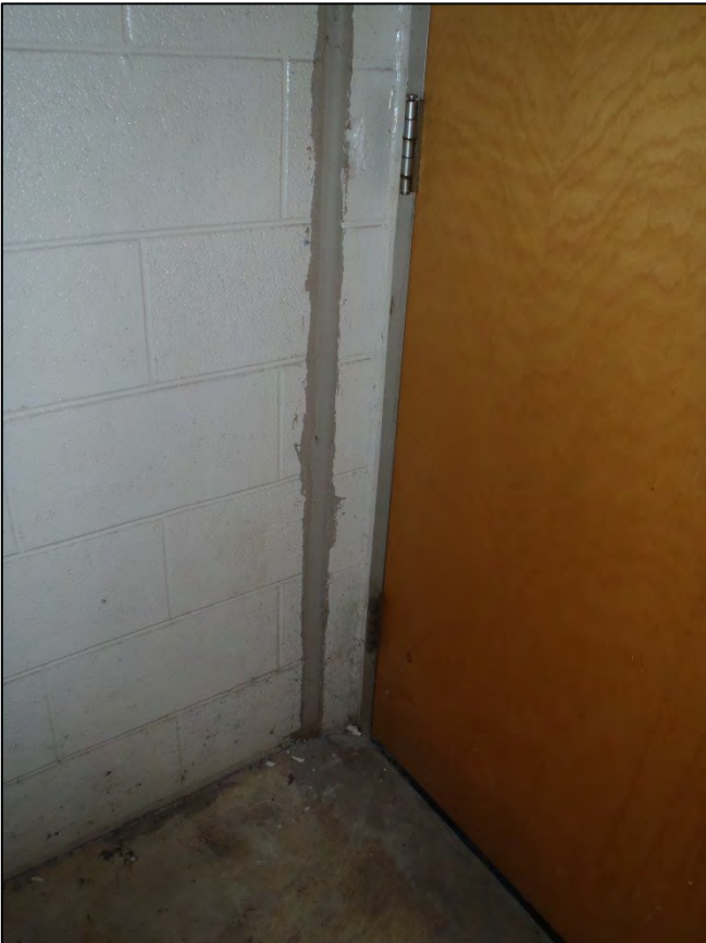
NO. 120 – FIRST FLOOR BASEMENT ADDITION – INTERIOR JOINT SEALANT
