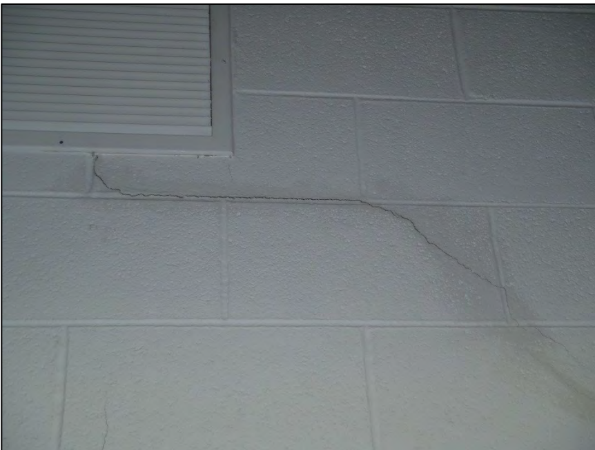
NO. 115 – FIRST FLOOR – INTERIOR CRACKS IN A CONCRETE MASONRY PARTITION WALL
