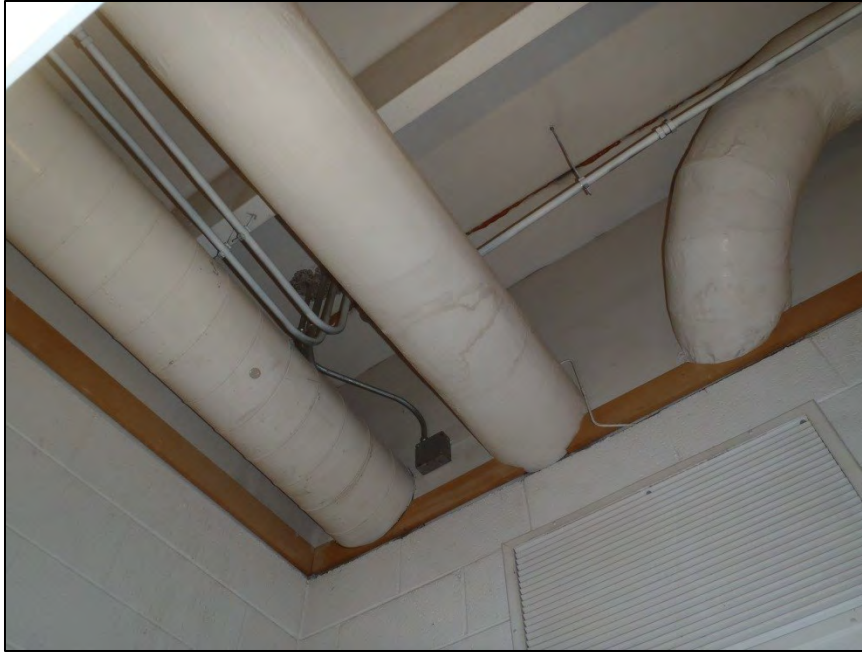
NO. 158 – SECOND FLOOR ROOM 221 – WATER STAINED DUCT WORK FROM WATER INFILTRATION AND/OR CONDENSATION
