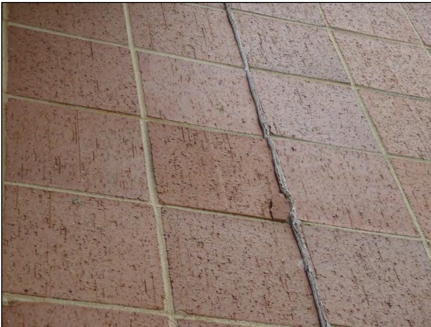
NO. 68 – NORTH ELEVATION ADJACENT TO THE CENTER EXTERIOR STAIRWELL – DETERIORATED JOINT SEALANT
