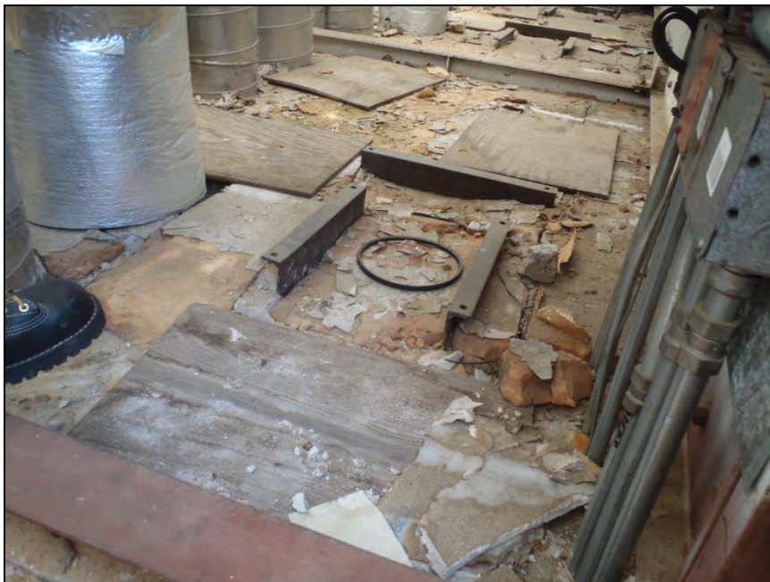
NO. 215 – ROOF SKYLIGHT/MECHANICAL ENCLOSURE – WATER DAMAGED INTERIOR FINISHES
