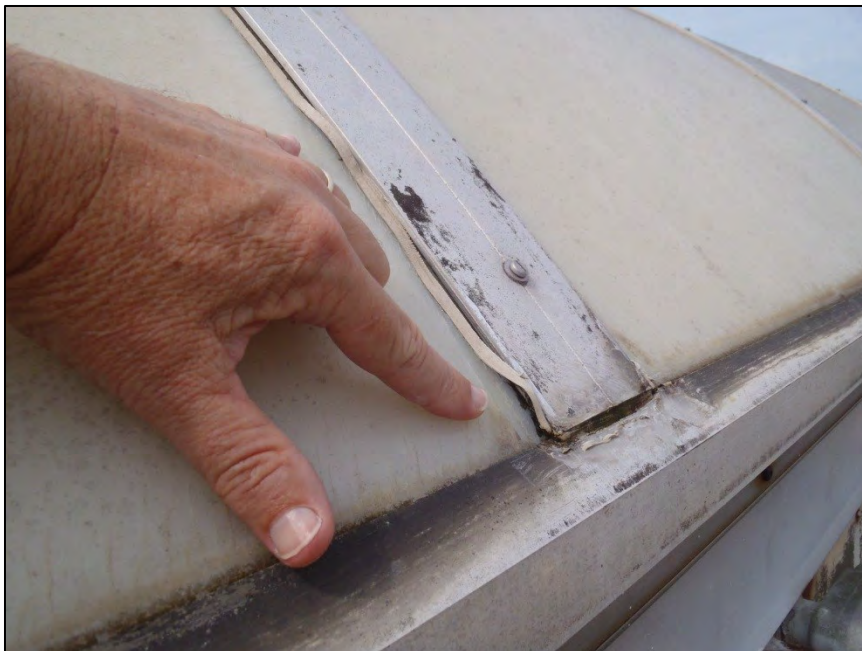
NO. 205 – ROOF SKYLIGHT/MECHANICAL ENCLOSURE – DETERIORATED JOINT SEALANTS ALLOWING WATER INFILTRATION
