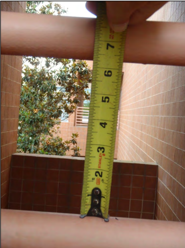
NO. 77 – NORTH ELEVATION AT WEST EXTERIOR STAIRWELL – INADEQUATE GUARDRAIL PICKET SPACINGS
