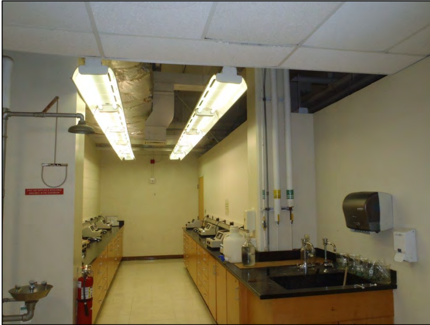
NO. 133 – SECOND FLOOR GENERAL CHEMISTRY LABORATORY 207 – MISSING CEILING TILES
