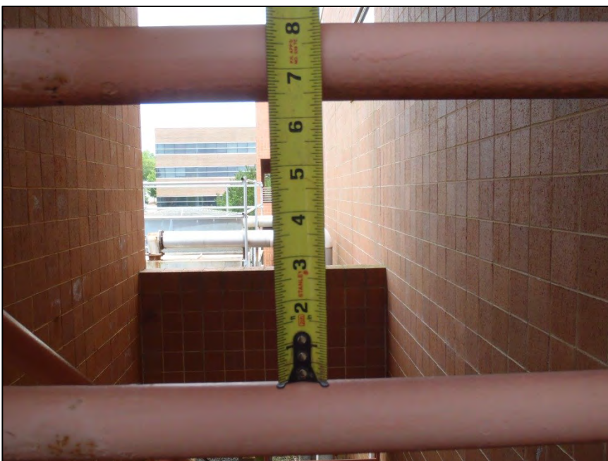
NO. 64 – NORTH ELEVATION AT CENTER EXTERIOR STAIRWELL – INADEQUATE GUARDRAIL PICKET SPACINGS
