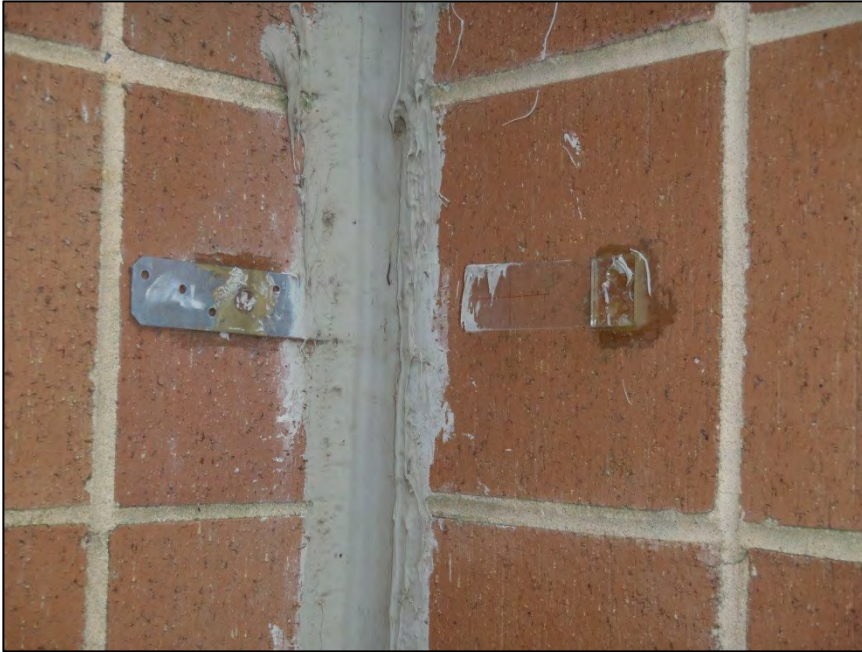
NO. 80 – WEST ELEVATION AT BASEMENT ADDITION – DETERIORATED JOINT SEALANT
