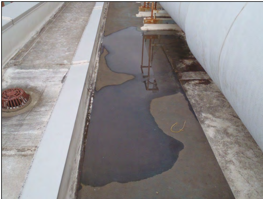
NO. 195 – ROOF – PONDING WATER
