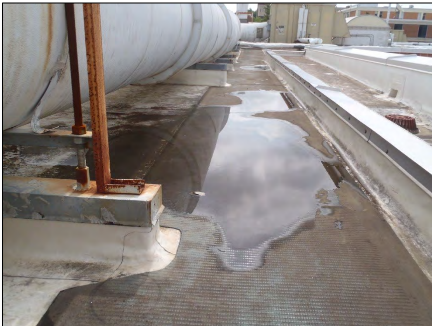
NO. 199 – ROOF – PONDING WATER
