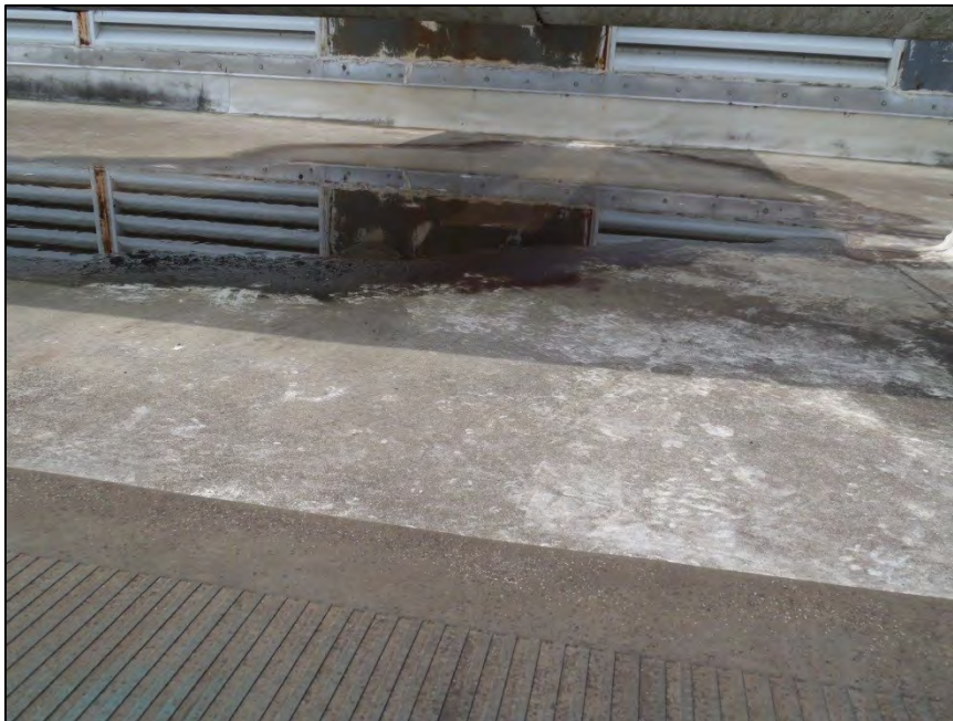
NO. 198 – ROOF – PONDING WATER
