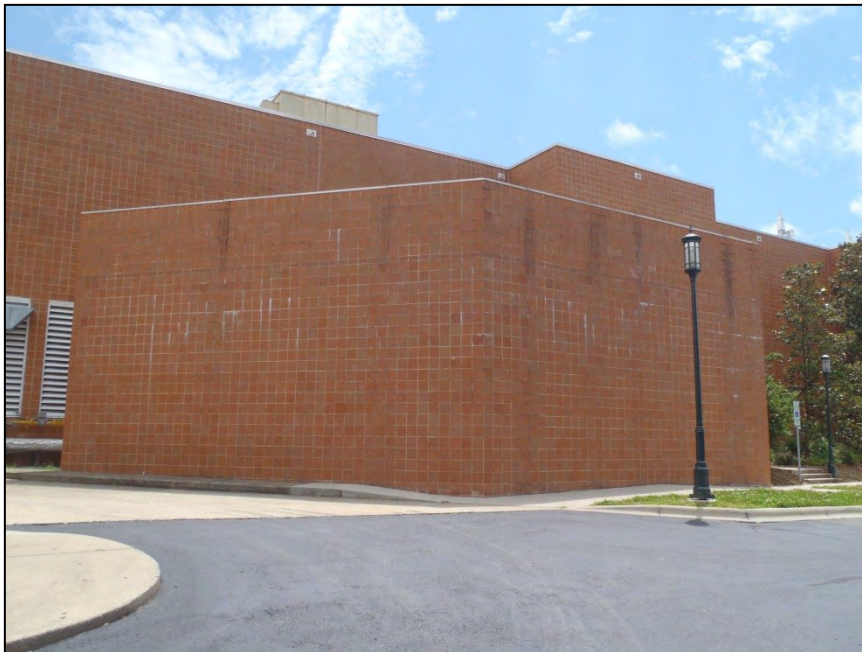
NO. 51 – NORTH ELEVATION AT EXTERIOR SCREEN WALL – EFFLORESCENCE AT EXTERIOR BRICK VENEER
