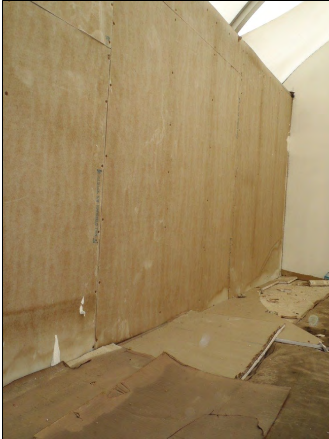
NO. 212 – ROOF SKYLIGHT/MECHANICAL ENCLOSURE – WATER DAMAGED INTERIOR FINISHES
