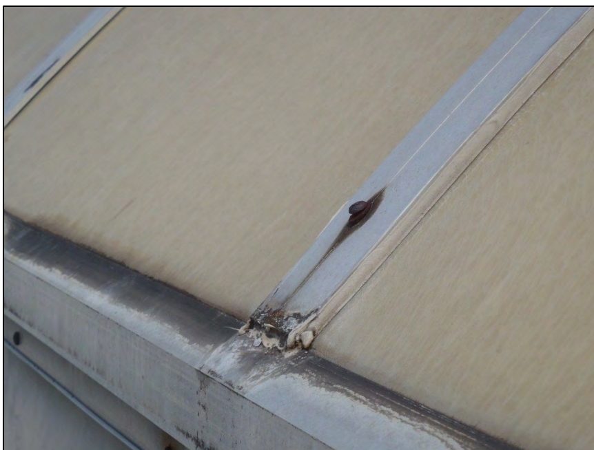
NO. 209 – ROOF SKYLIGHT/MECHANICAL ENCLOSURE – LOOSE FRAMING ALLOWING WATER INFILTRATION
