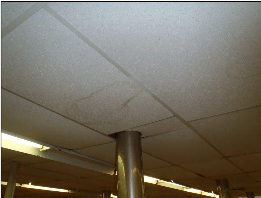
NO. 128 – SECOND FLOOR GENERAL CHEMISTRY LABORATORY 207 – DAMAGED CEILING TILES FROM WATER INFILTRATION
