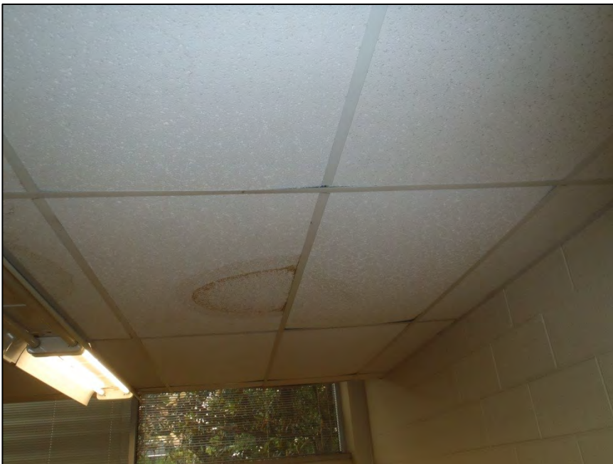
NO. 129 – SECOND FLOOR GENERAL CHEMISTRY LABORATORY 207 – DAMAGED CEILING TILES FROM WATER INFILTRATION
