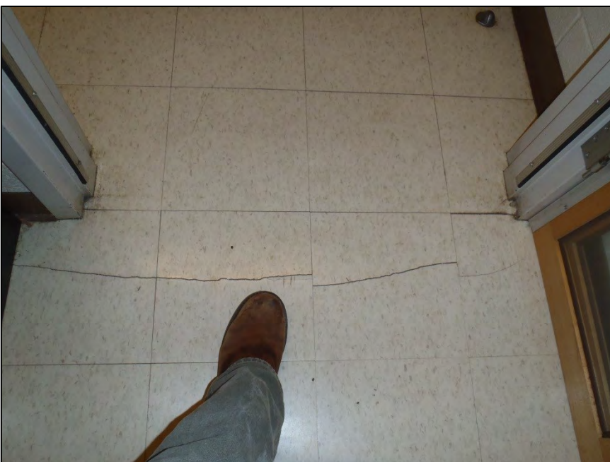
NO. 116 – FIRST FLOOR – CRACKED INTERIOR FLOOR FINISHES
