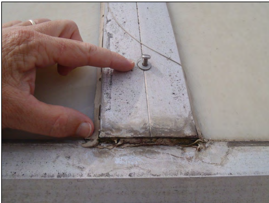
NO. 208 – ROOF SKYLIGHT/MECHANICAL ENCLOSURE – LOOSE FRAMING ALLOWING WATER INFILTRATION
