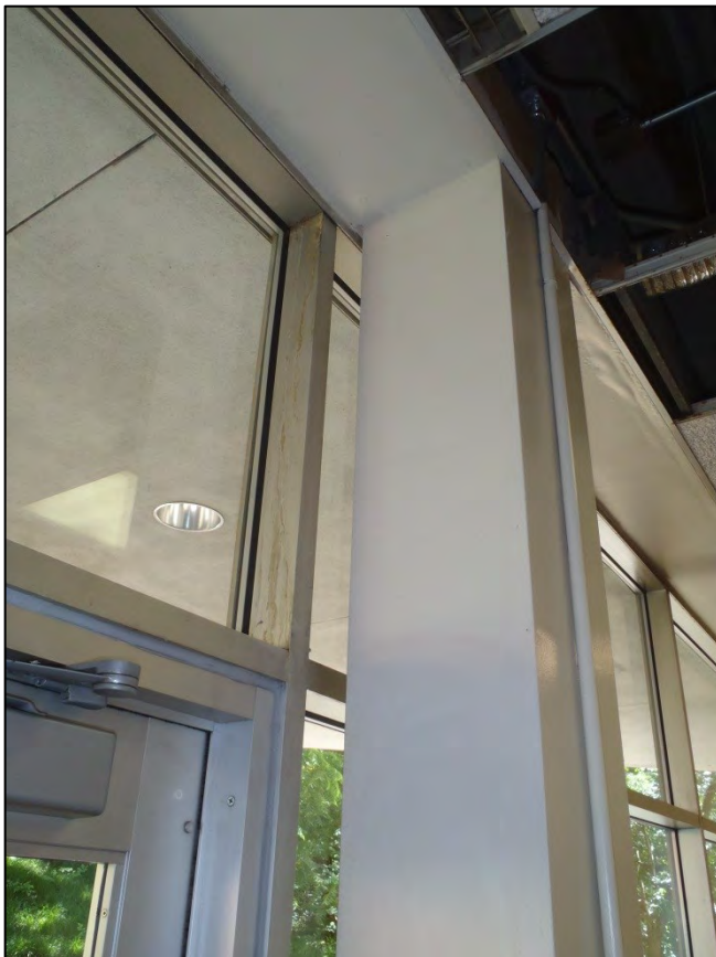
NO. 102 – FIRST FLOOR AT SOUTHEAST ENTRY PLAZA – WATER INFILTRATION
