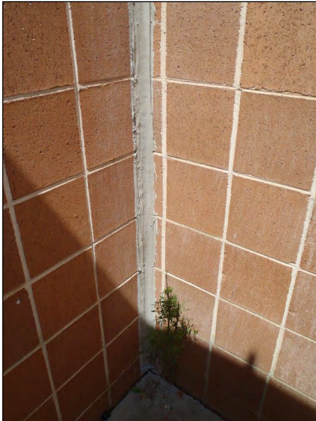
NO. 83 – WEST ELEVATION AT BASEMENT ADDITION – DETERIORATED JOINT SEALANT
