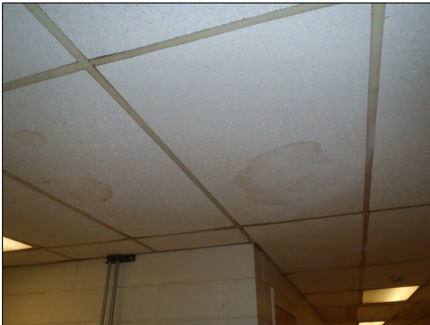
NO. 153 – SECOND FLOOR CORRIDOR – WATER DAMAGED CEILING TILES FROM WATER INFILTRATION
