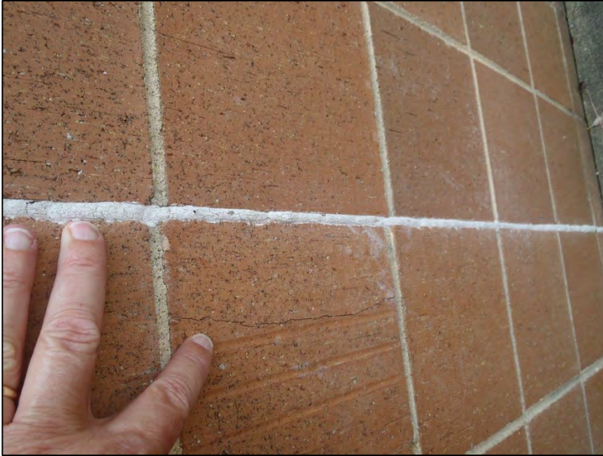
NO. 67 – NORTH ELEVATION ADJACENT TO THE CENTER EXTERIOR STAIRWELL – DETERIORATED JOINT SEALANT AND CRACKED INDIVIDUAL BRICK MASONRY UNIT
