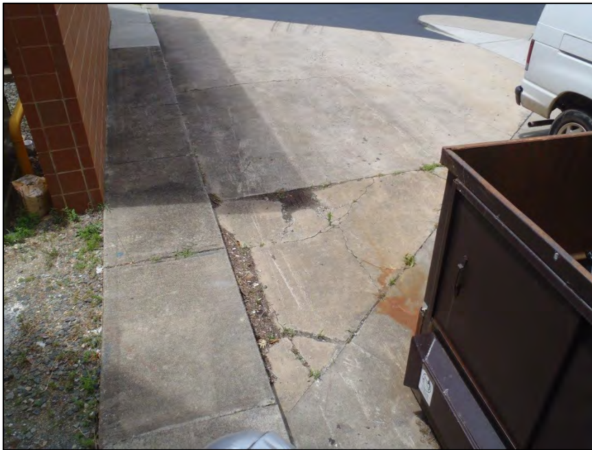
NO. 48 – NORTH ELEVATION AT LOADING DOCK – DETERIORATED EXTERIOR CONCRETE SLAB
