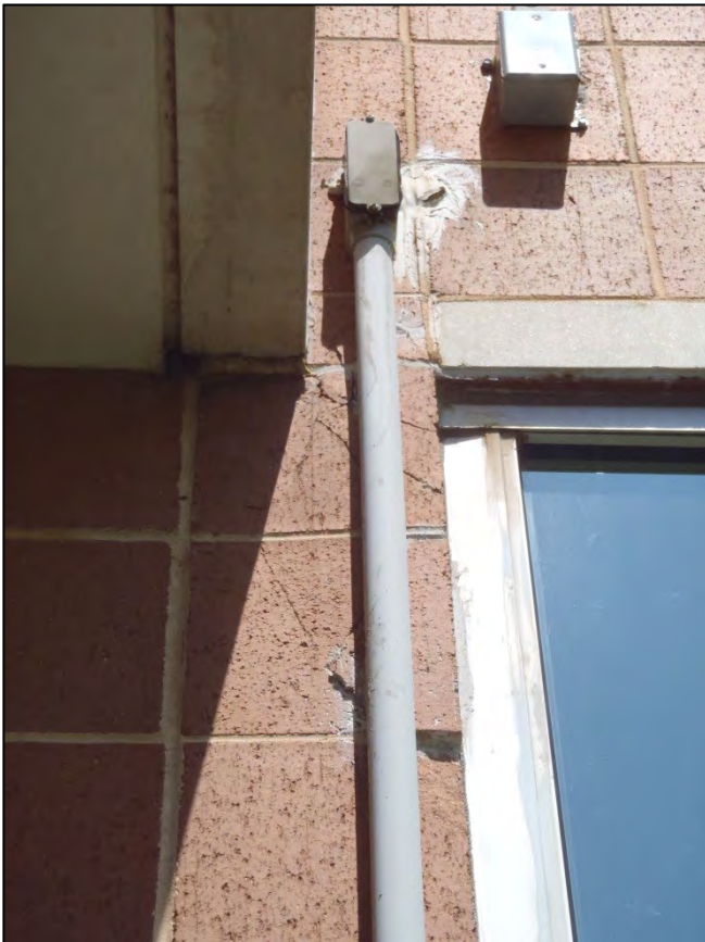
NO. 89 – SOUTHWEST ELEVATION – CRACKED INDIVIDUAL BRICK MASONRY UNITS
