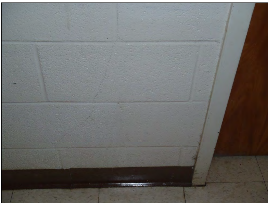
NO. 113 – FIRST FLOOR INTERIOR HALLWAY – CRACKED INDIVIDUAL CONCRETE MASONRY UNIT
