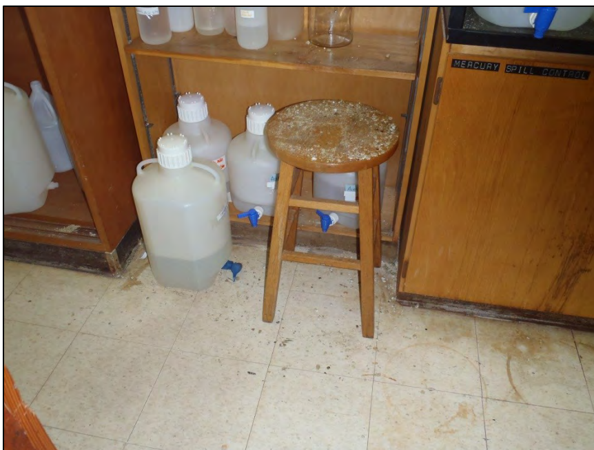
NO. 162 – SECOND FLOOR ROOM 225A – CHEMICALLY STAINED FURNITURE AND FLOOR FINISHES
