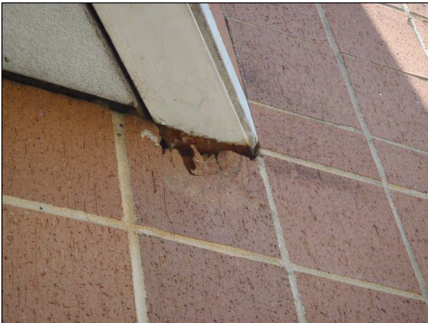
NO. 32 – SOUTHEAST ELEVATION AT MAIN ENTRANCE – CRACKED BRICK VENEER AT GIRDER BEARING
