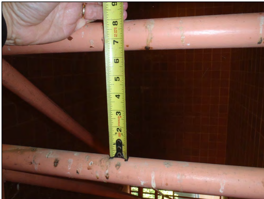
NO. 45 – NORTH ELEVATION AT EAST EXTERIOR STAIRWELL – INADEQUATE GUARDRAIL PICKET SPACINGS
