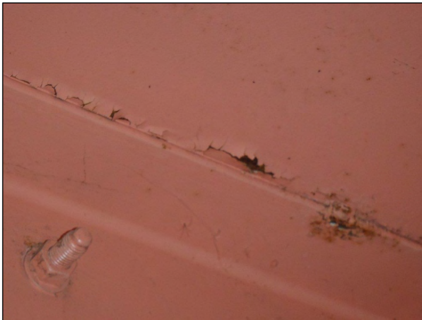
NO. 60 – NORTH ELEVATION AT CENTER EXTERIOR STAIRWELL – DETERIORATED LANDING FRAMING
