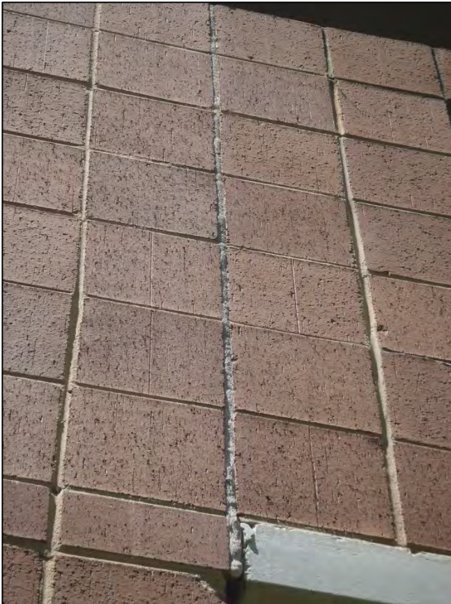
NO. 96 – SOUTH ELEVATION – DETERIORATED JOINT SEALANT
