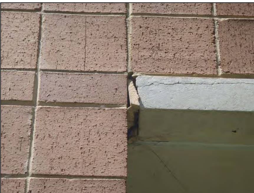
NO. 94 – SOUTH ELEVATION – DETERIORATED JOINT REQUIRING JOINT SEALANT
