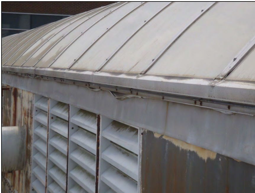
NO. 204 – ROOF SKYLIGHT/MECHANICAL ENCLOSURE – DETERIORATED JOINT SEALANTS ALLOWING WATER INFILTRATION
