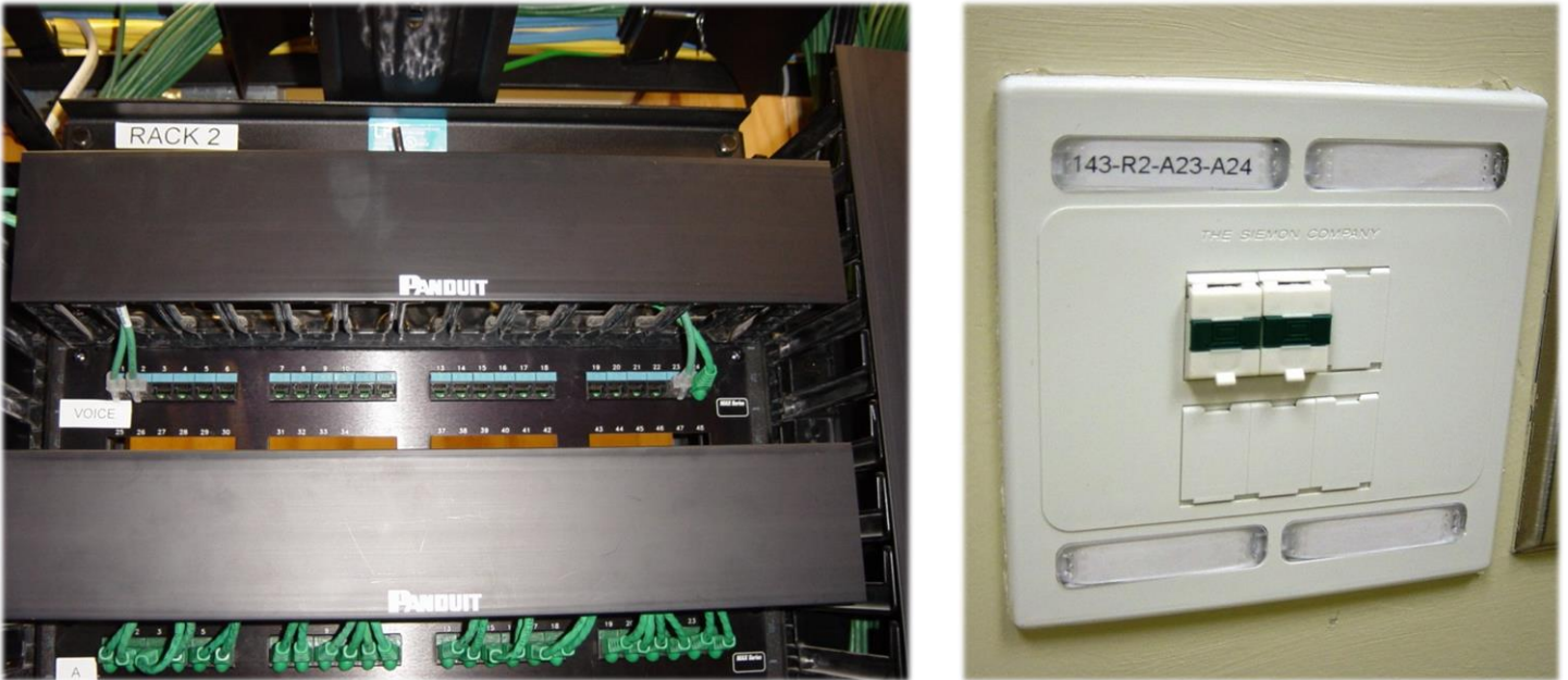
Figure 8: From the patch panel to the end user, UNCC ITS utilizes a standard for colored icons to identify the port function on the faceplate. Specific university functions will dictate which termination method or hardware is used to protect the network ports and will be determined during project design.
