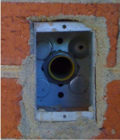
Exterior door swipe Belden 8732 control wire
