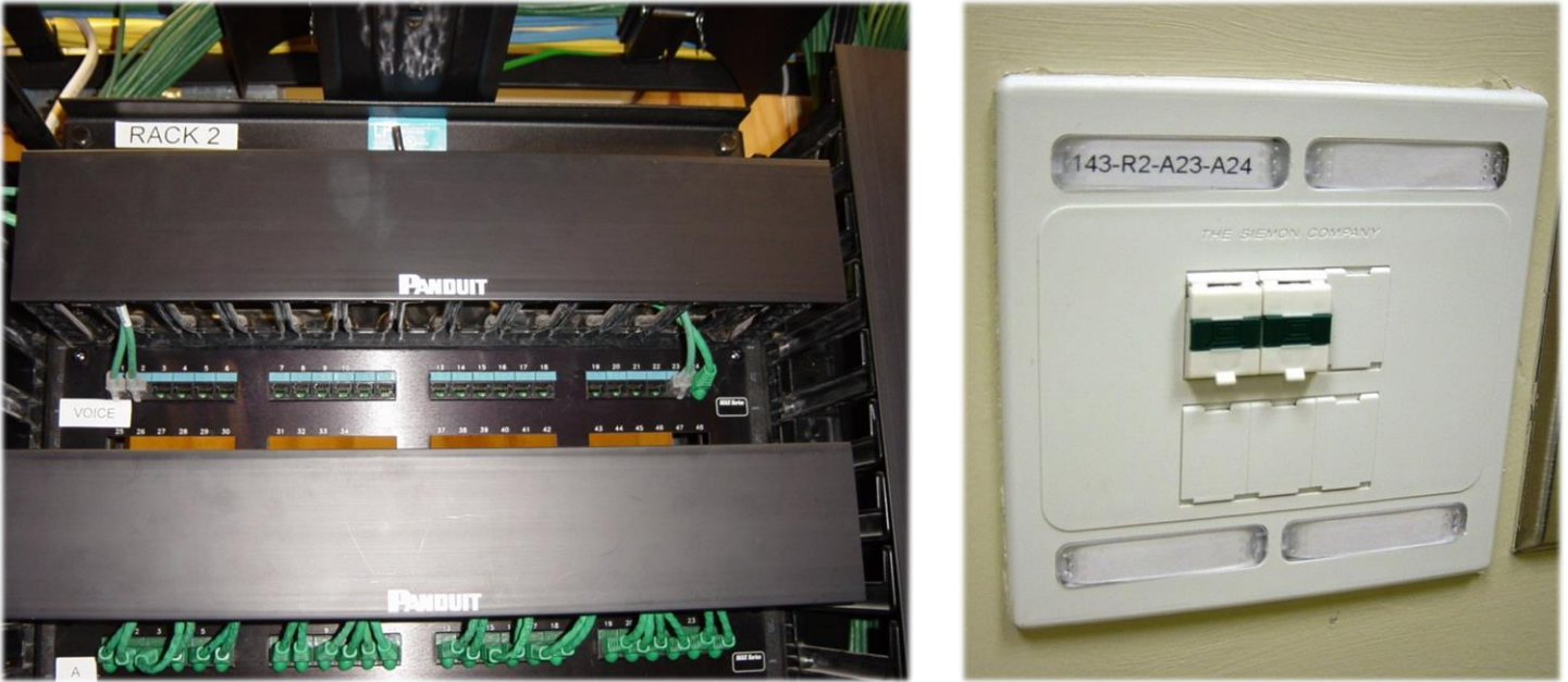
Figure 8: From the patch panel to the end user, UNCC ITS utilizes a standard for colored icons to identify the port function on the faceplate. Specific university functions will dictate which termination method or hardware is used to protect the network ports and will be determined during project design.
